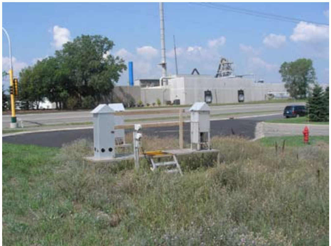
Air monitoring equipment near Gopher Resources, a lead recycling facility in Dakota County
