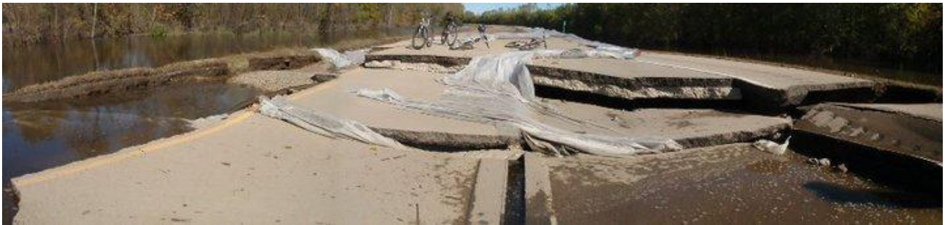
Flash flooding in September 2010 caused Highway 169 to break apart north of St. Peter.
