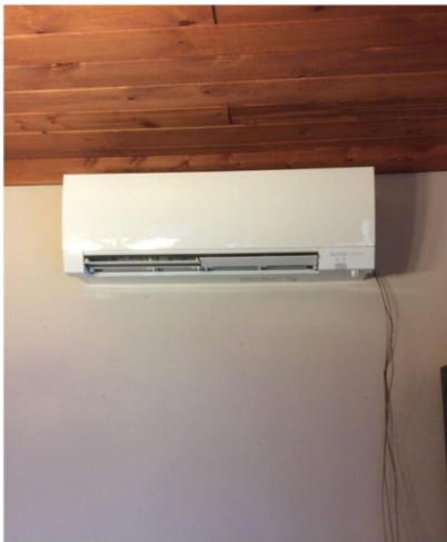
Cold climate ductless mini-split air source heat pump
