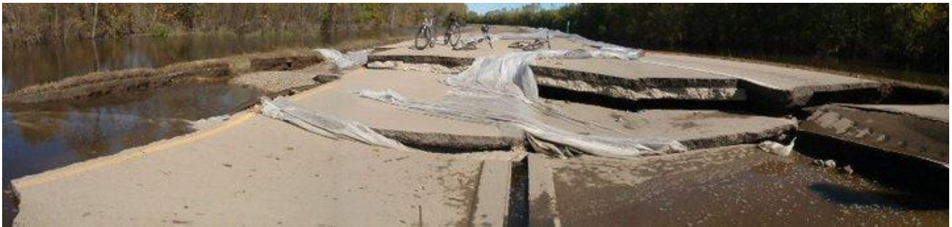
Flash flooding in September 2010 caused Highway 169 to break apart north of St. Peter.
