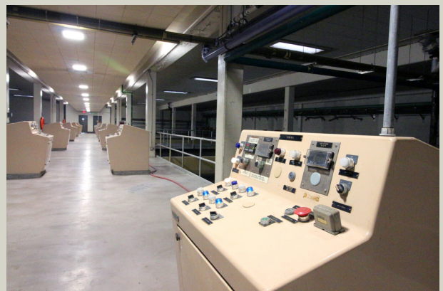
Control panels original to 1978 still exist for the effluent filters.
