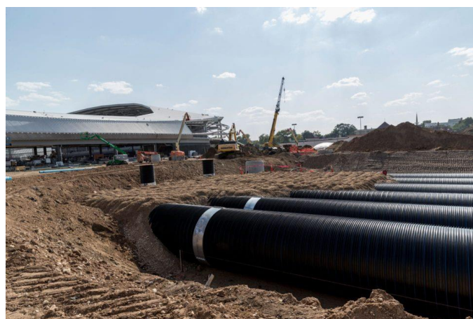
Figure 2: Stormwater Reuse at Allianz Field
