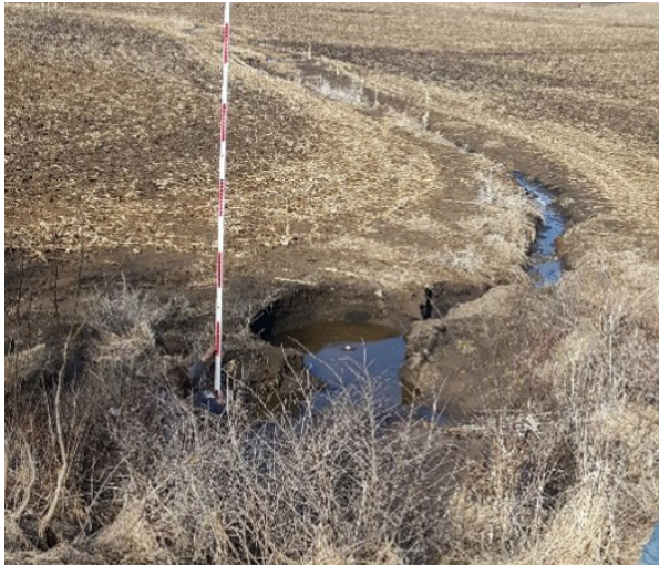
Site in need of a grade stabilization structure and a grassed waterway prior to construction
