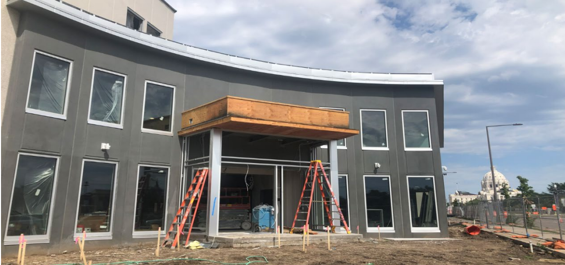
Photo of St. Paul City School under construction along University Avenue. CAAPB worked closely with school leadership and architects on planning, design, and approval. (Credit: Peter Musty)
