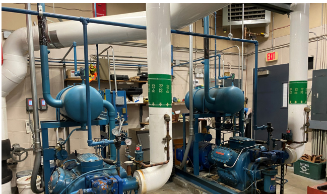
CURRENT REFRIGERATION SYSTEM
