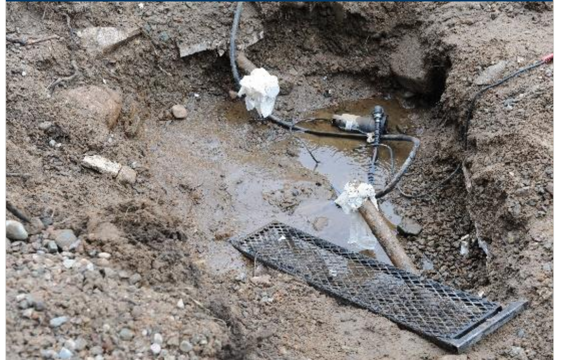
Damaged underground pipes
