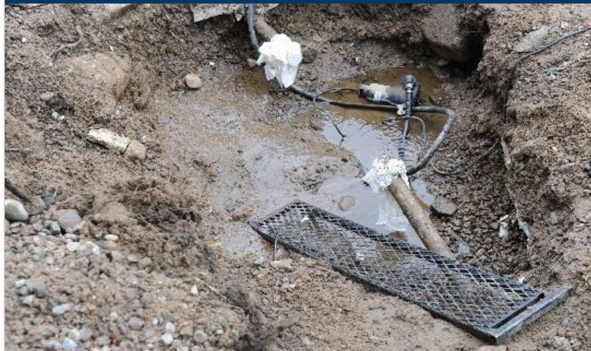
Damaged underground pipes
