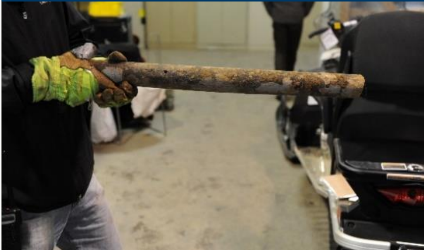
Corroded and deteriorating water line pipes
