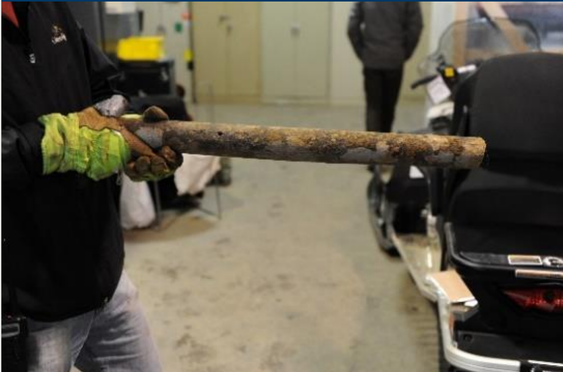
Corroded and deteriorating water line pipes
