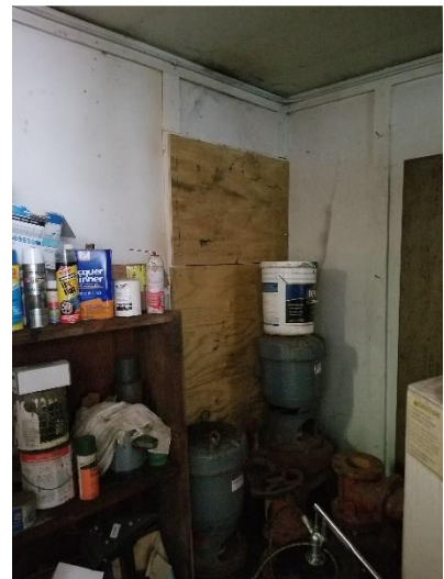
Backdoor boarded due to vandalism and decay
