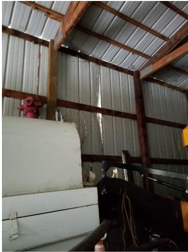
Hole in the side of the building
