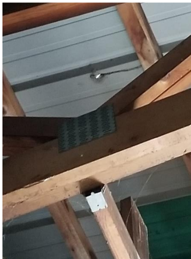
Hole in ceiling
