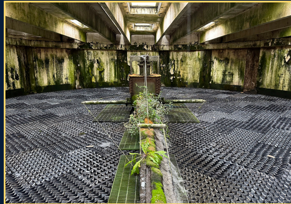
The interior of the trickling filters is failing, with distribution arms that no longer rotate within the deteriorating concrete structure.
