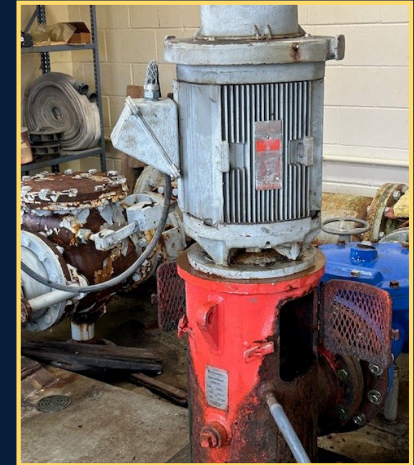
Old trickling filter pump and motor that feeds trickling filter. Pump and piping in need of repair.
