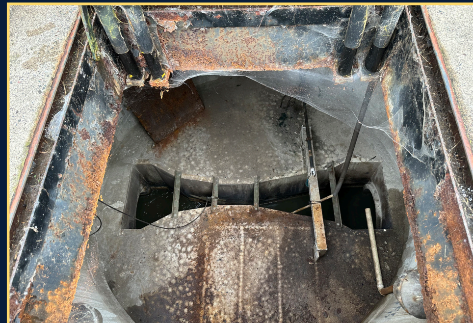
All wastewater flows through this flume for monitoring, but the concrete is deteriorating with exposed rebar.
