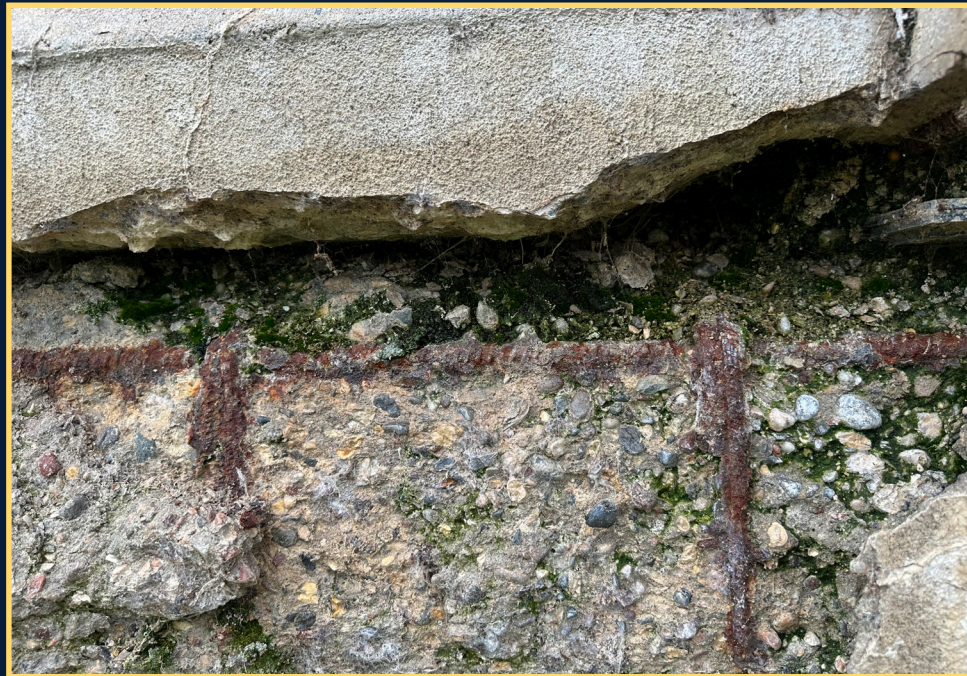
The two trickling filters have deteriorating concrete structures with exposed rebar.
