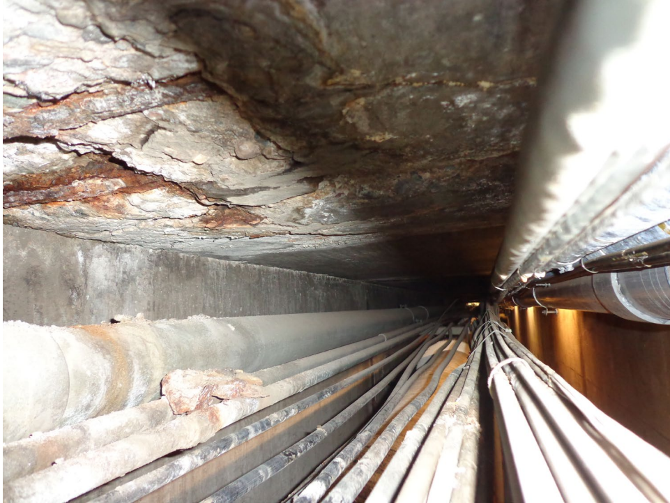
Crumbling Utility Tunnels
