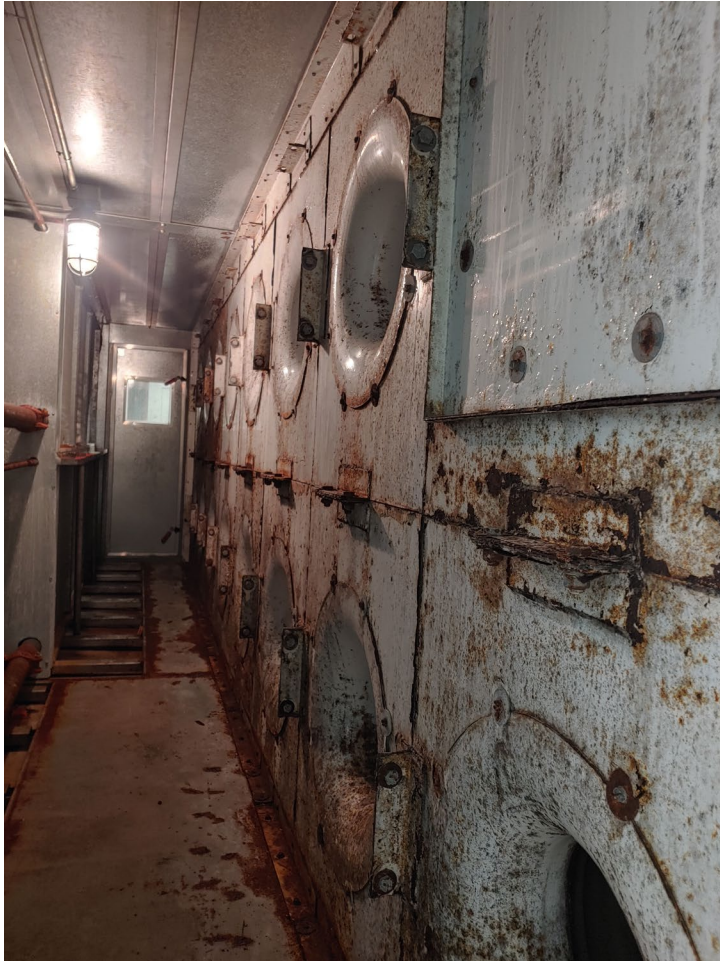
Obsolete HVAC Equipment
