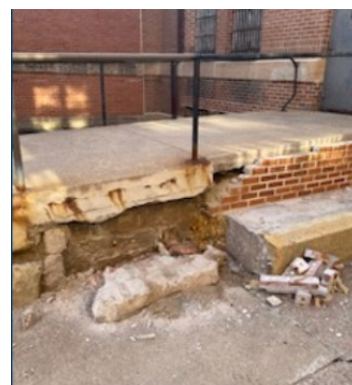
ADA entrance ramp crumbling apart
