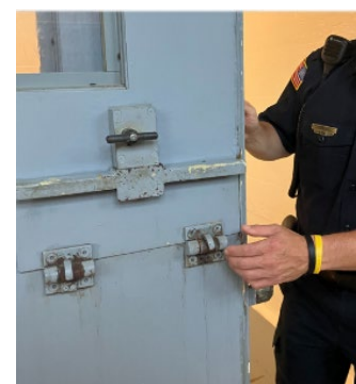
Rusting manual locks on cells
