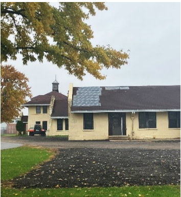
Heavily used building with roof in crisis condition
