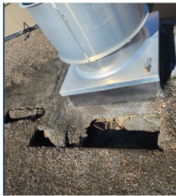
Hole in roof at Stillwater causing massive leaks
