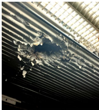
Hole in ceiling that is continuously growing
