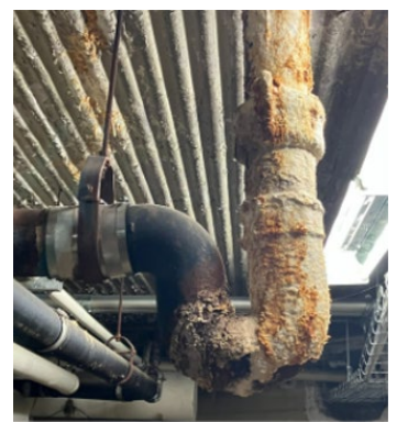
Corroding water pipes
