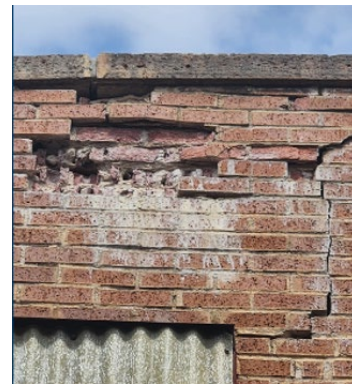
Crumbling brick in outside walls
