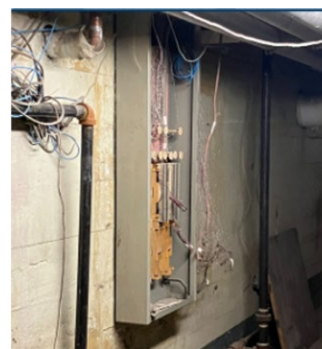
Exposed and outdated electrical wiring
