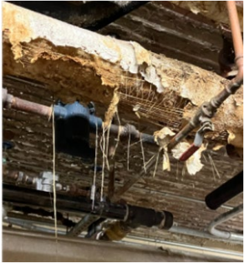
Deteriorating pipes and vents
