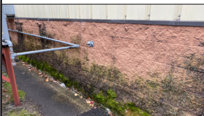
Mold caused by moisture & drainage issues
