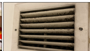
Aging HVAC systems cause air quality & health concerns
