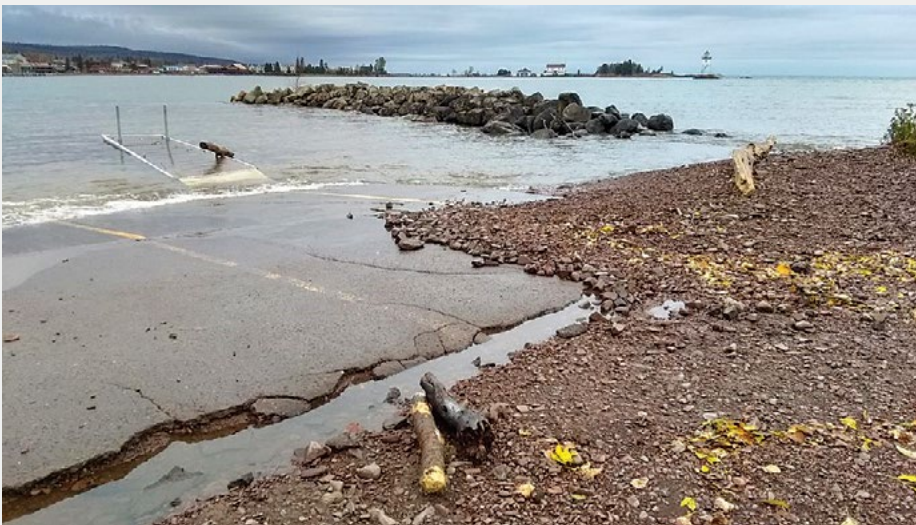
Left: The Grand Marais water access and breakwater in failed condition.
