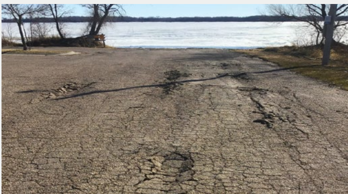
German Lake PWA showing failure of the asphalt pavement. This pavement must be completely replaced.
