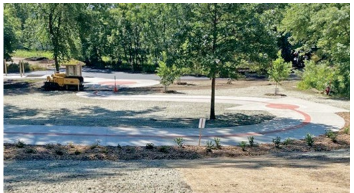
Newly-reconstructed walkway to the visitor center at Fort Snelling State Park. The previous walkway did not meet ADA slope standards.
