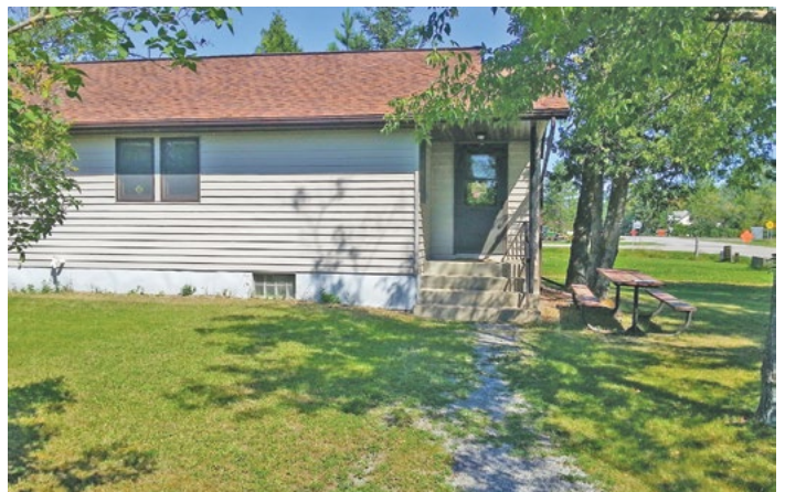
Public entrance of Williams Forestry office. Sidewalk and stairs do not meet ADA requirements.
