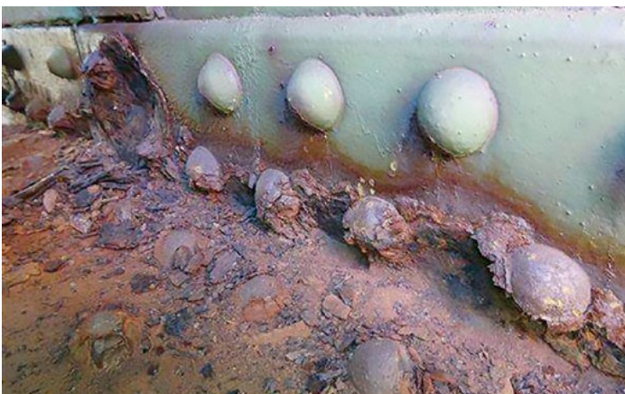
Photo at left: Extremely corroded structural steel on the bridge at Tettegouche State Park.
