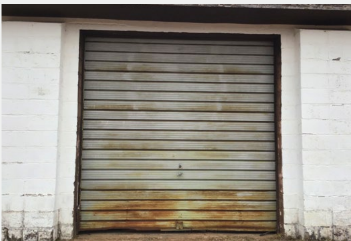
General Andrews Forestry area office garage. The metal overhead door is severely corroded and must be replaced.
