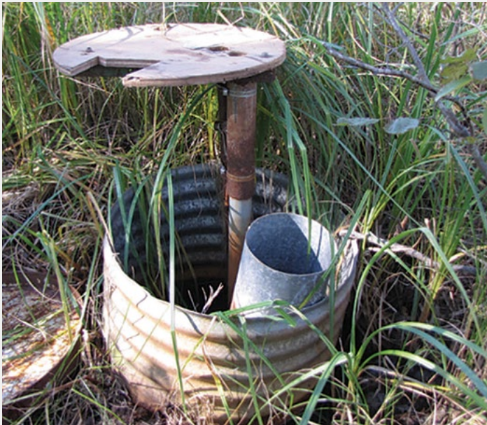
Monitoring well on state forest land in Aitkin County in poor condition.
