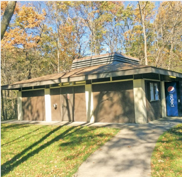
The old Cedar Hill Campground shower building at Whitewater State Park. This building was in poor condition, undersized, energy inefficient, and did not meet the needs of today's campers.
