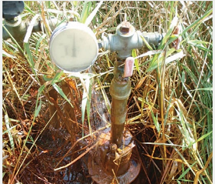
Monitoring well in need of replacement.
