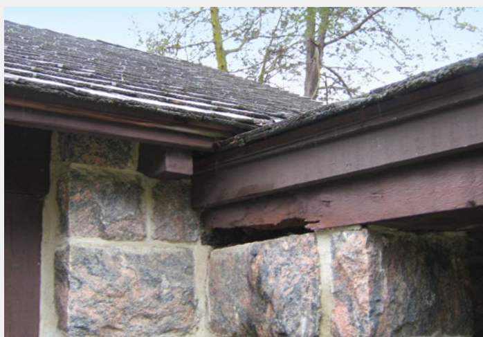
Fort Ridgely State Park campground picnic shelter with rotting supporting timbers.
