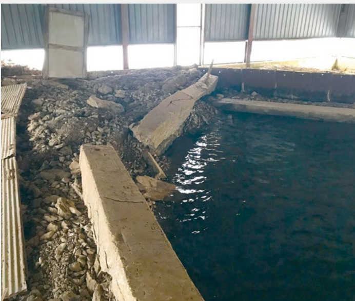
Lanesboro Hatchery dilapidated spring pool wall.
