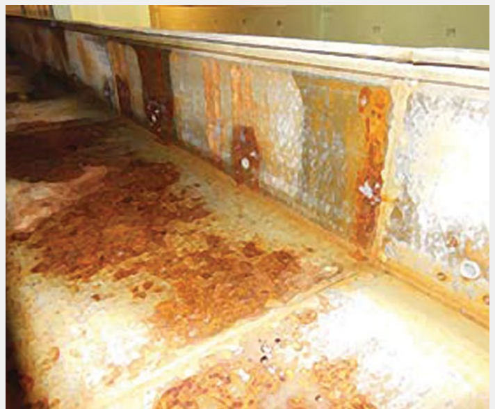
Waterville Hatchery fry tank in poor condition.
