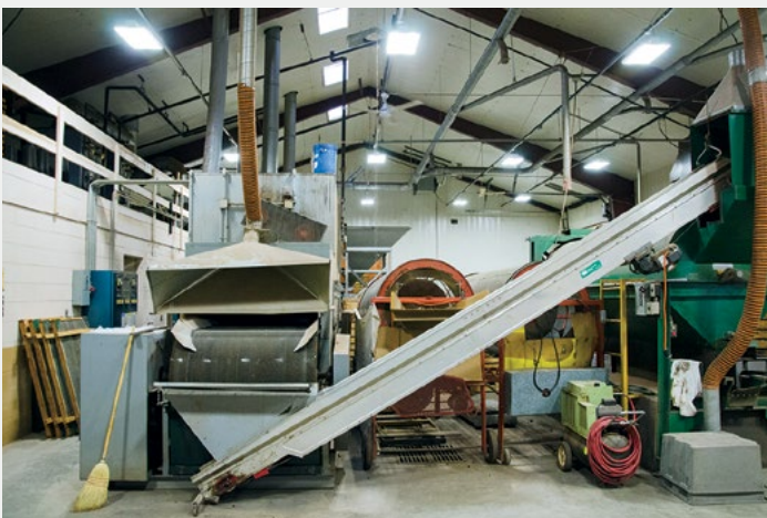
The pine cone seed extractor. The equipment in the seed extractor is old, no longer maintainable, and must be replaced with modern, efficient equipment. The facility’s HVAC and dust controls also require replacement.
