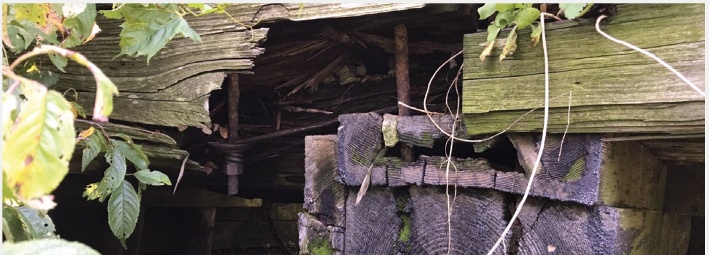
Below: Wild Indigo Prairie SNA. This trail bridge is in imminent danger of collapse due to rotting structural timbers. This bridge must be completely replaced; it is not repairable.
