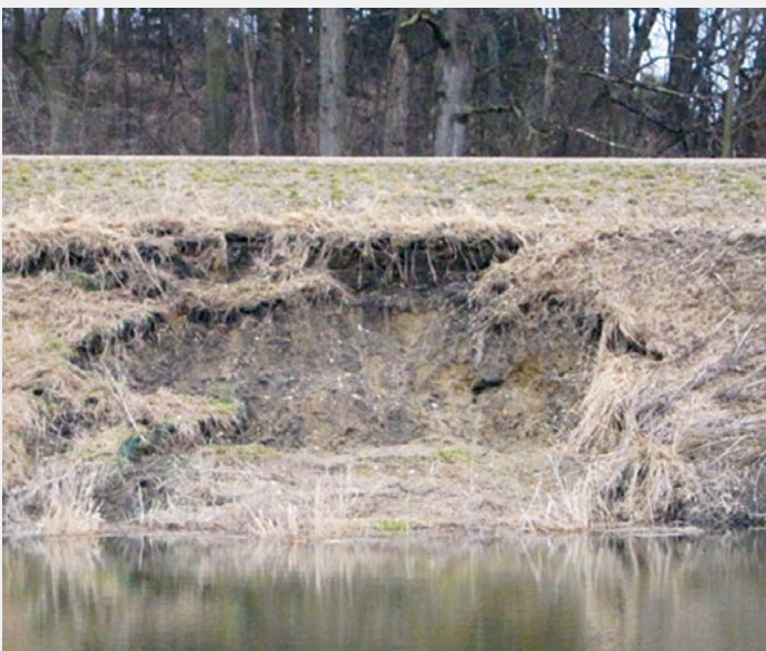
Failing pond dike at Waterville Hatchery.
