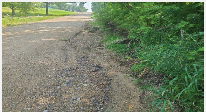
Lake Rachel PWA gravel road showing ongoing storm water erosion. This area must be repaired or erosion will get worse.
