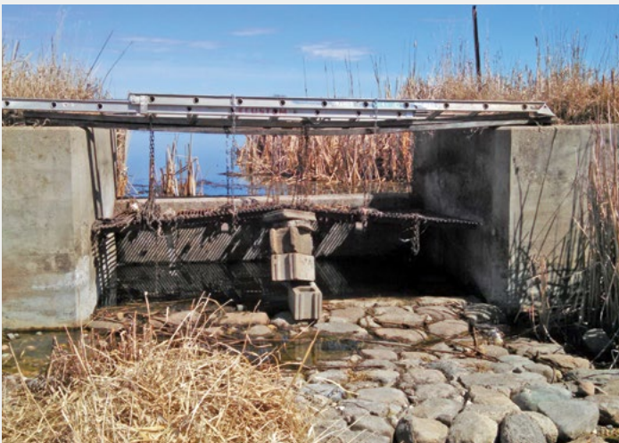
Silver Lake (Sibley County) water control structure in crisis condition. Note the control gate is held up by a stack of cinder blocks. A replacement for this structure is currently in design.
