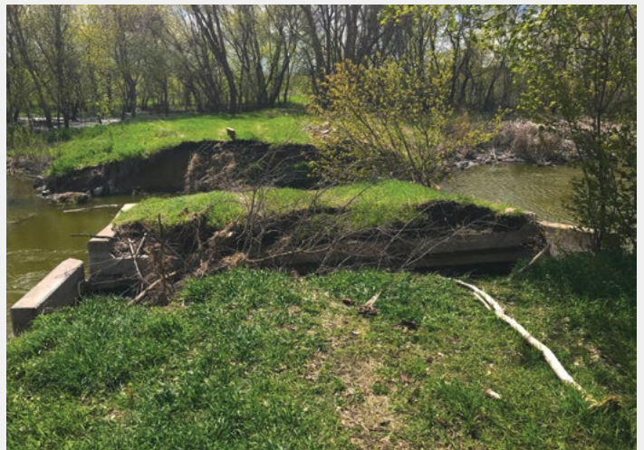
Perkins Lake water control structure failure. The earth embankment washed out and lake levels can no longer be managed.
