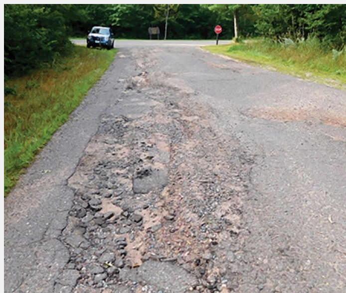
Wild River State Park. This asphalt road has failed and requires full reconstruction.
