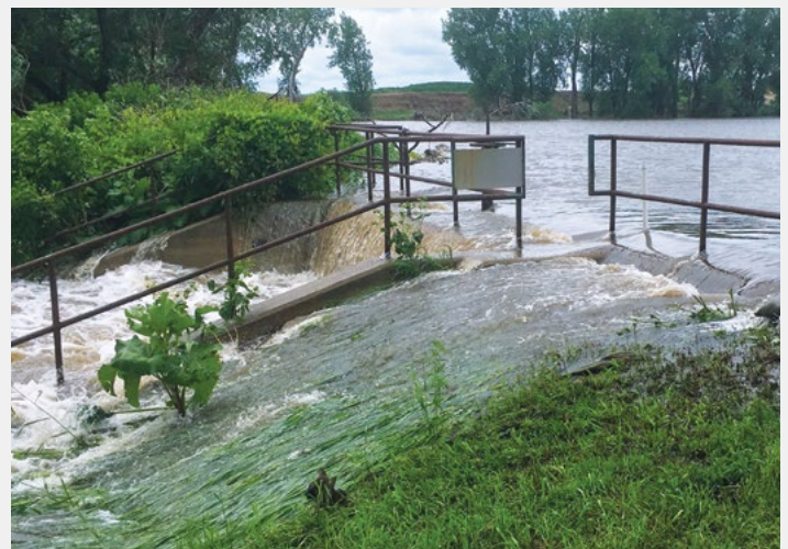
Warren Lake dam failure caused by overtopping. The spillway is undersized to safely pass incoming floodwaters.
