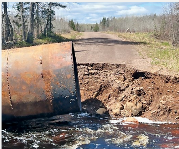
This very large culvert on a forest system road in Finland State Forest was washed out by a storm in 2022. Storm events are steadily increasing in intensity, overwhelming old road infrastructure that was not designed for today’s climate.
