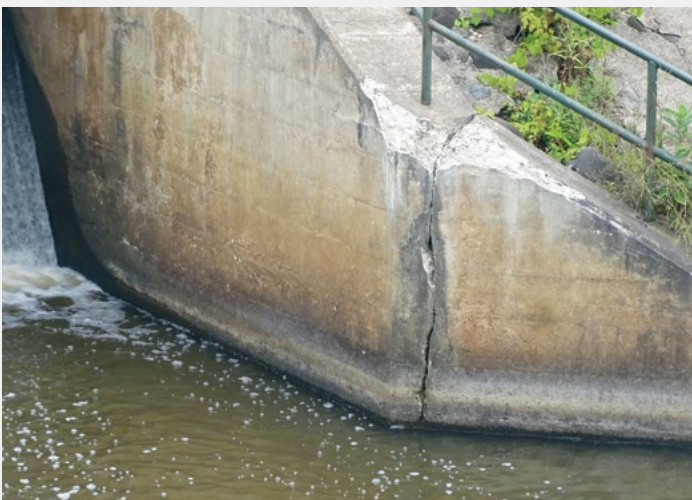
A wing wall of the Grindstone Dam spillway. The concrete is cracked completely through, increasing the likelihood of collapse and subsequent failure of the dam.
