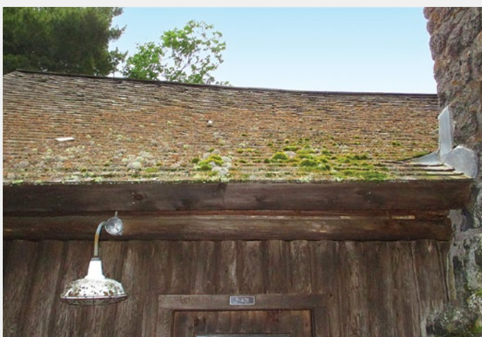
Tettegouche State Park historic camp lodge roof in crisis condition.
