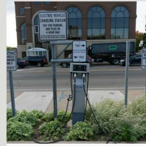
State Fleet Electric Vehicle Charging Infrastructure
