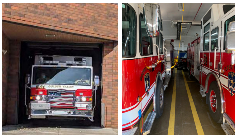
Apparatus bays doors are undersized for modern equipment, making for difficult entry and exit while responding to calls.
