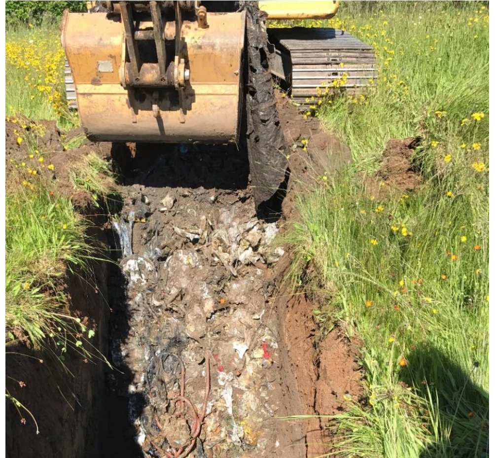
Brookston Landfill lacks adequate cover and other environmental controls to protect human health and the environment.
