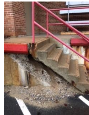
Crumbling loading dock stairway at AMRTC
