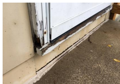
Rotting threshold on a state-operated group home serving clients with disabilities
