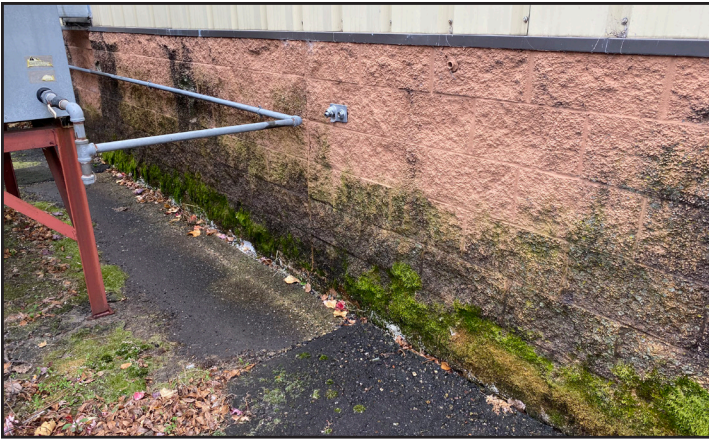
Mold is present on the exterior of the building due to moisture and drainage issues.
