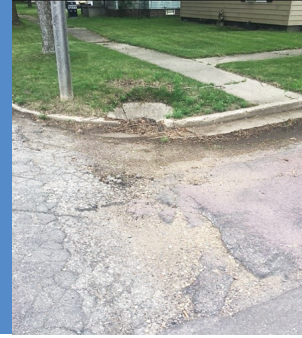
A deteriorated Storm Sewer Drain in Revere, MN
