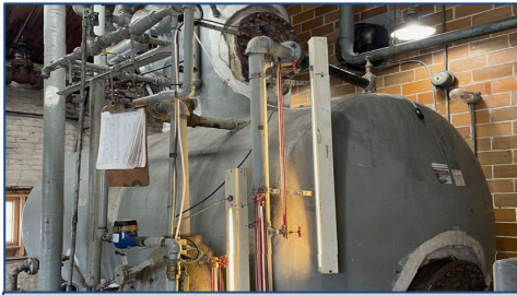
Heating Plant, UMC
