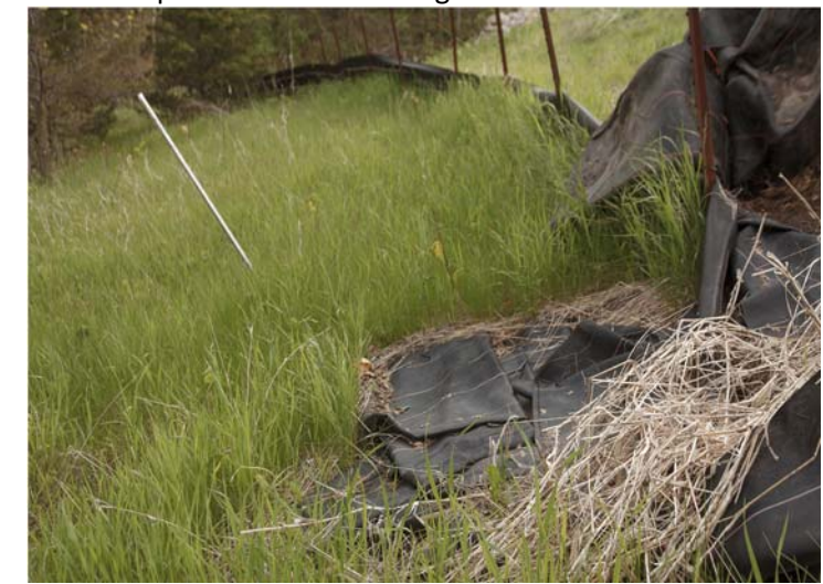
Silt fence products remains long after the need
