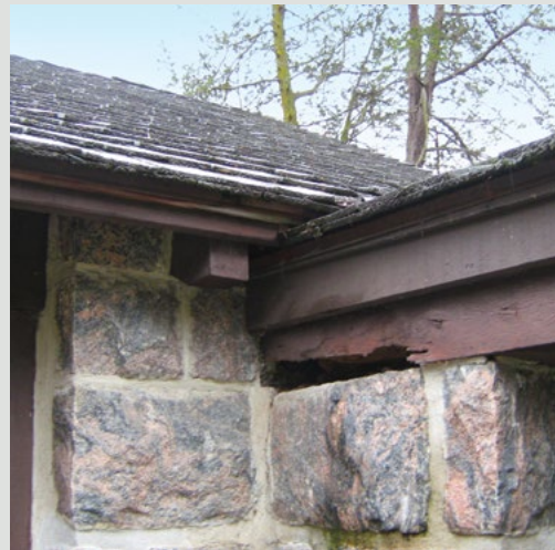
Fort Ridgely State Park campground picnic shelter with rotting supporting timbers.
