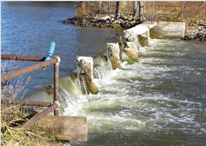
High Island Lake dam failure.
