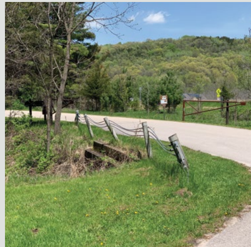
Whitewater State Park Cedar Hills campground guard rail failure.
