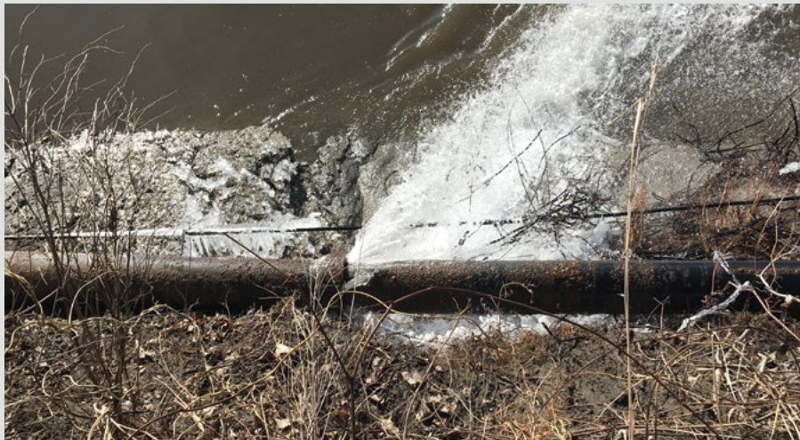
Water main break.
