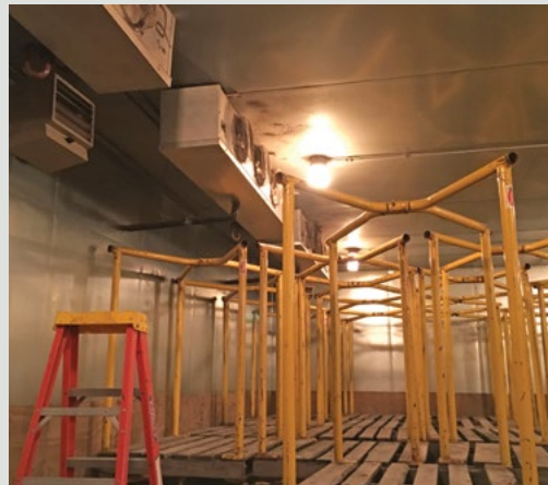
Pack house cooler in poor condition.
