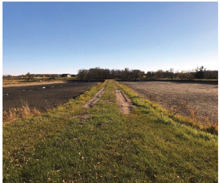
Failing dike road at New London Hatchery.
