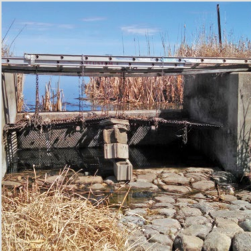
Silver Lake, LeSueur County, water control structure in crisis condition.
