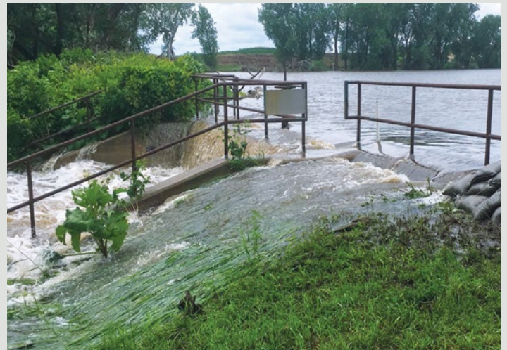
Warren Lake dam failure.
