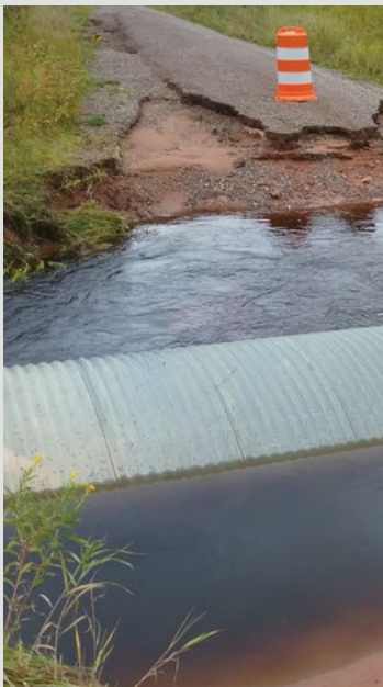
Harlis Forestry road washout damage.
