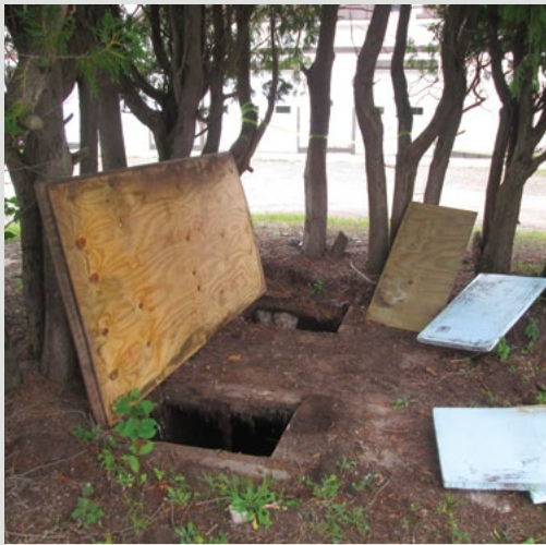
Septic holding tanks area poor condition prior to repair.
