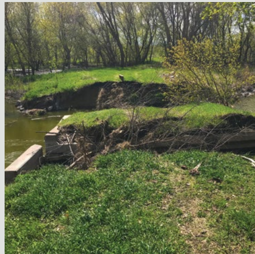
Perkins Lake water control structure failure.
