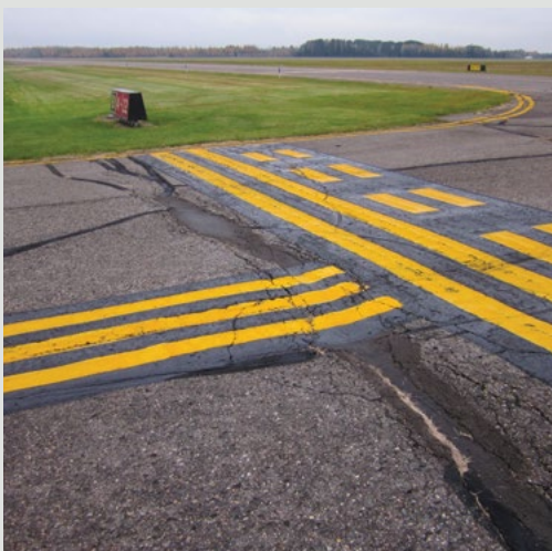
Hibbing air tanker base ramp in crisis condition.
