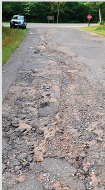
Wild River State Park road deterioration.
