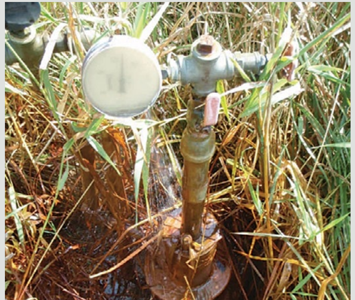
Monitoring well in need of replacement.
