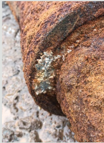
Septic piping poor condition prior to repair.
