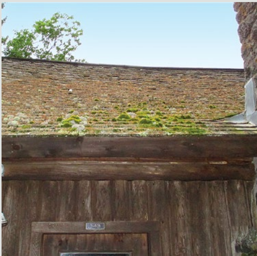
Tettegouche State Park historic camp lodge roof in crisis condition.
