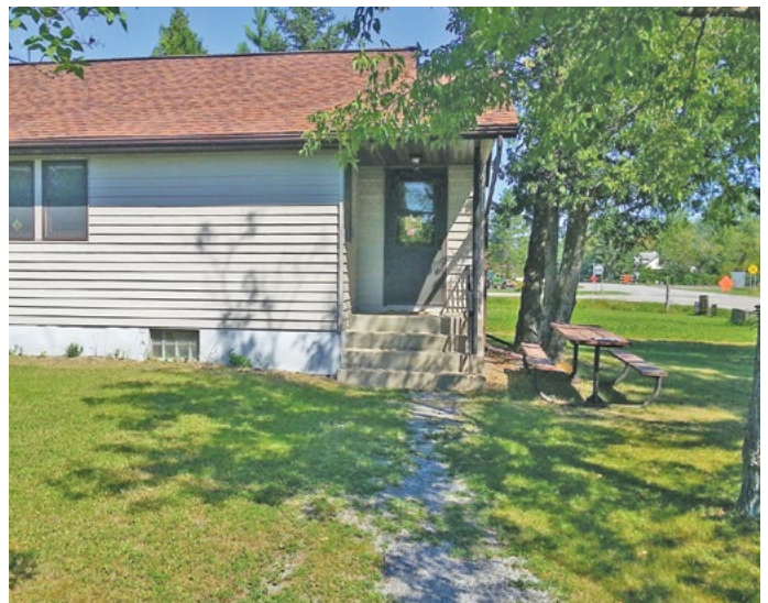
Public entrance of Williams Forestry office. Sidewalk and stairs do not meet ADA requirements.
