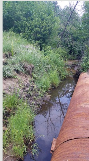
Trails culvert washout.
