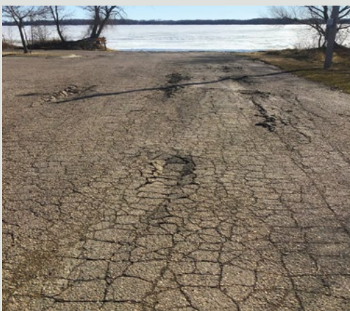
German Lake PWA pavement repair needs.
