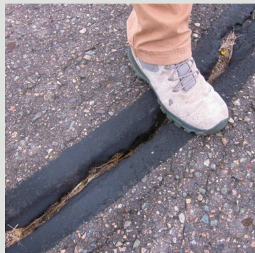
This deep crack at the Hibbing air tanker base ramp is unsafe for taxiing aircraft.
