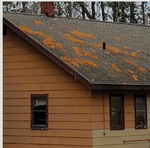
The Zimmerman Forestry Office is rated as "crisis" condition.
