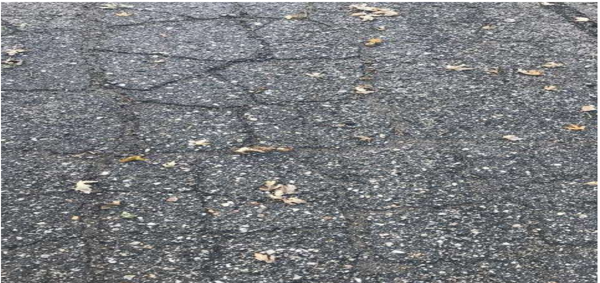
Closer up view of the cracks in the street.
