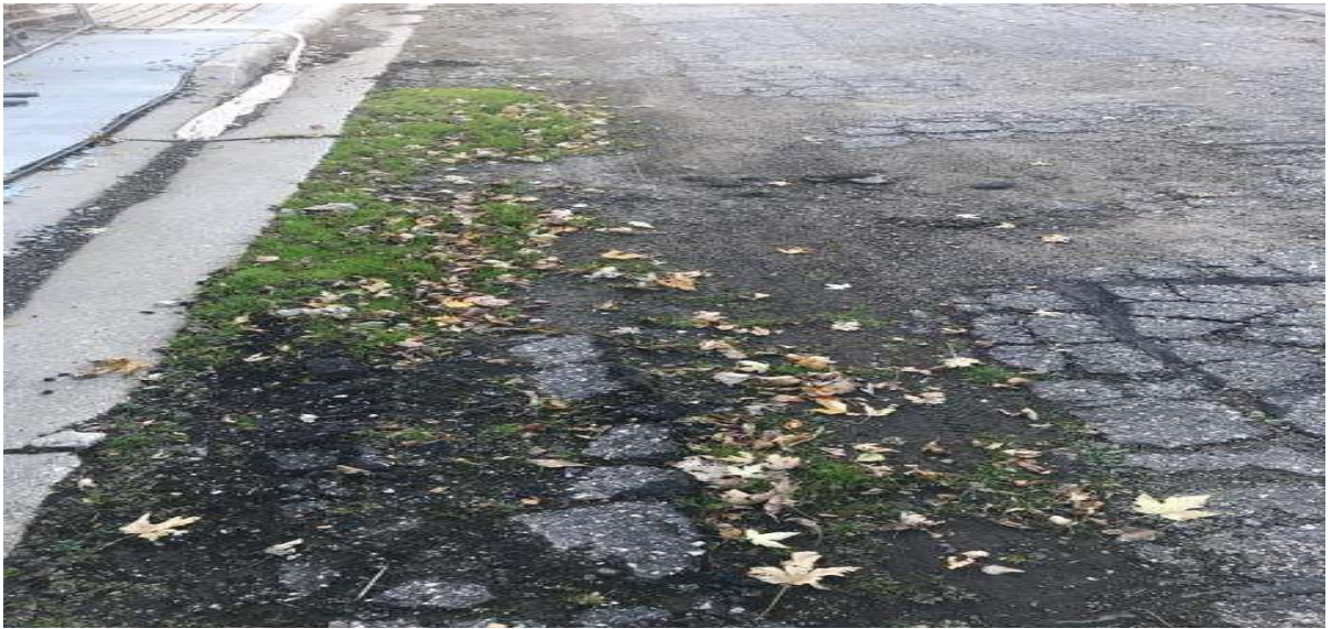
Above picture shows grass growing right up the cracks in the street.
