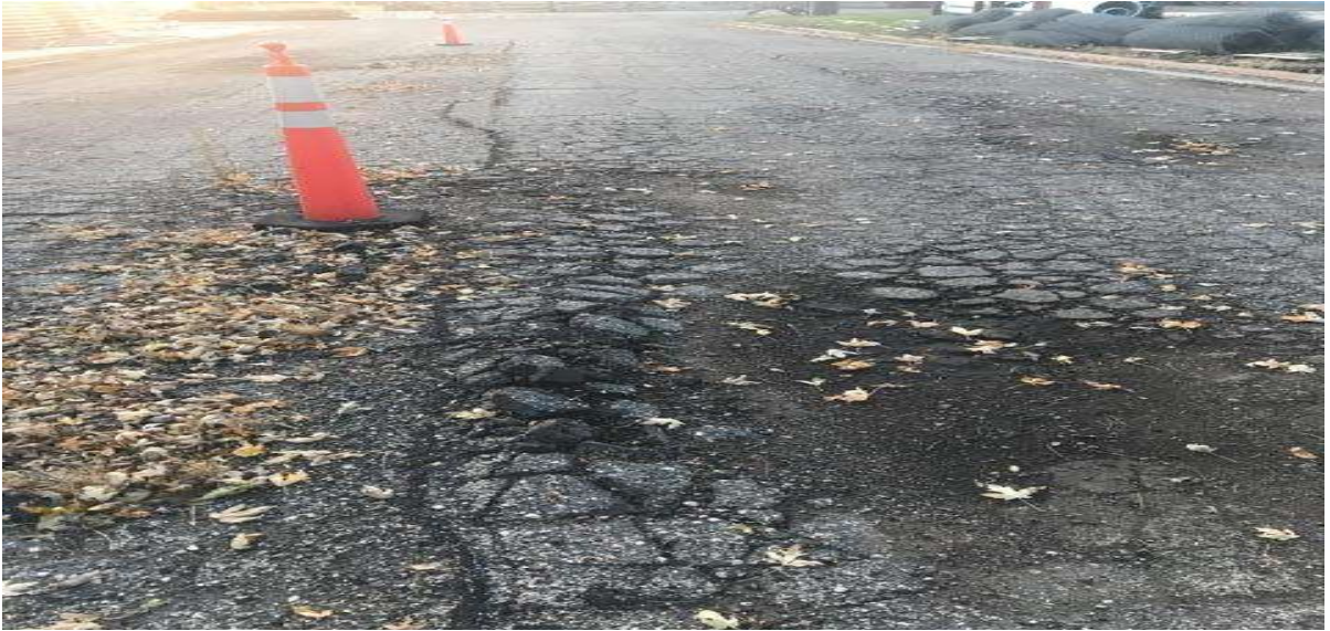
Closer view of the cracks in the street that are blocked off by cones so no traffic drives on it to prevent further damage to the street.
