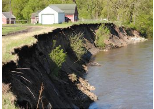
Bank failure on the Le Sueur River
