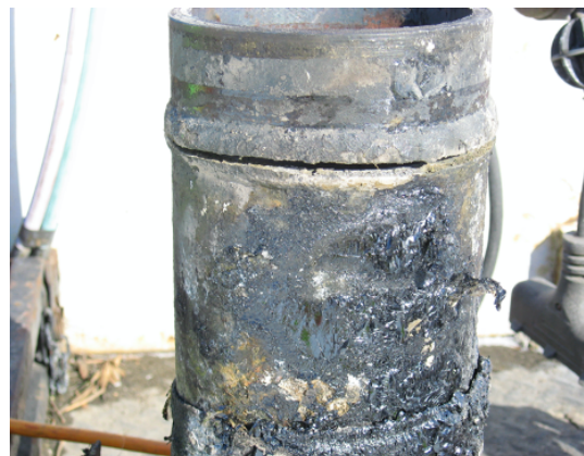
UM-Crookston Ruptured Natural Gas Main
