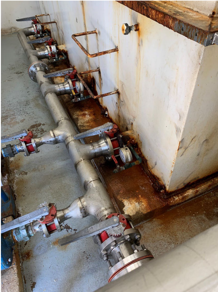
Figure 2 Severe corrosion and leaking from bottom corner
