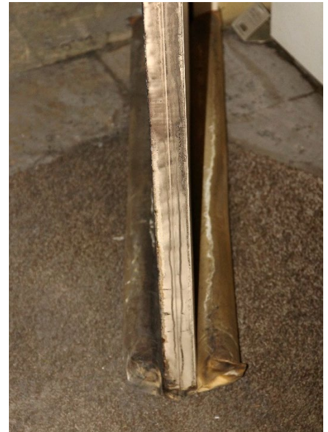
Figure 9: Seal under door of adjacent apartment
