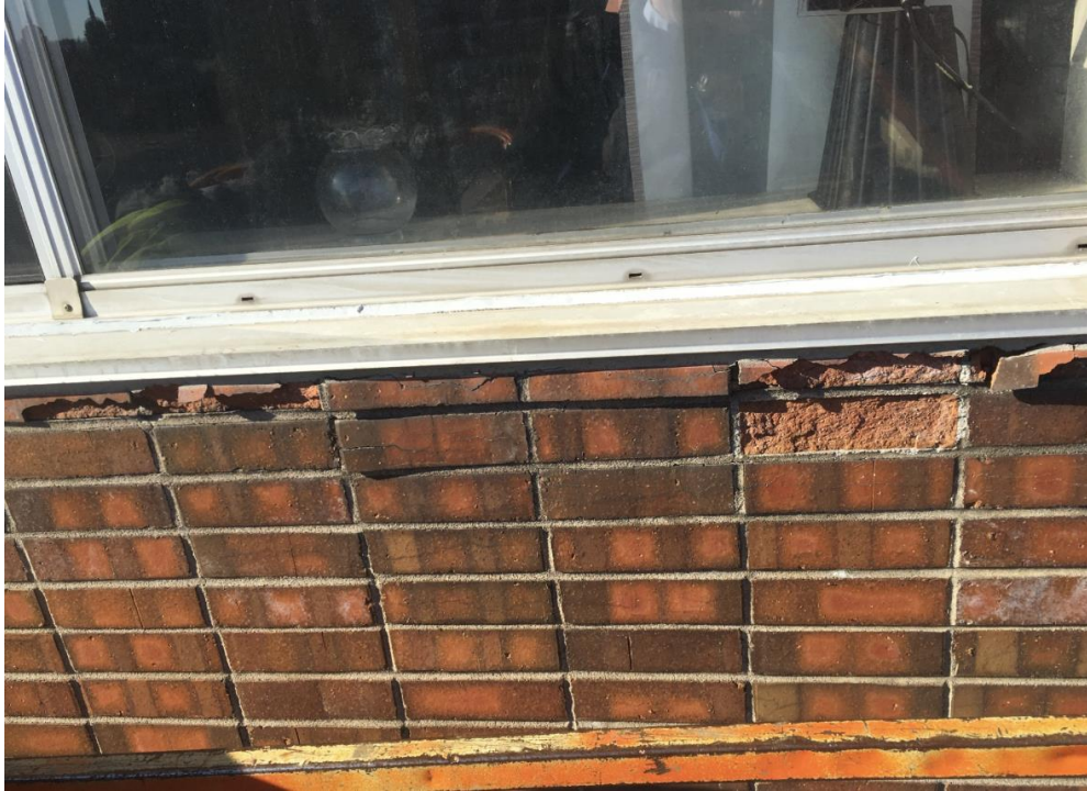
Bricks crumbling from façade and falling to sidewalks below.
