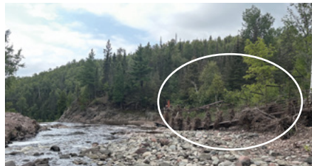
BEFORE: Tettegouche State Park High Falls Bridge washed out, June 2024.
