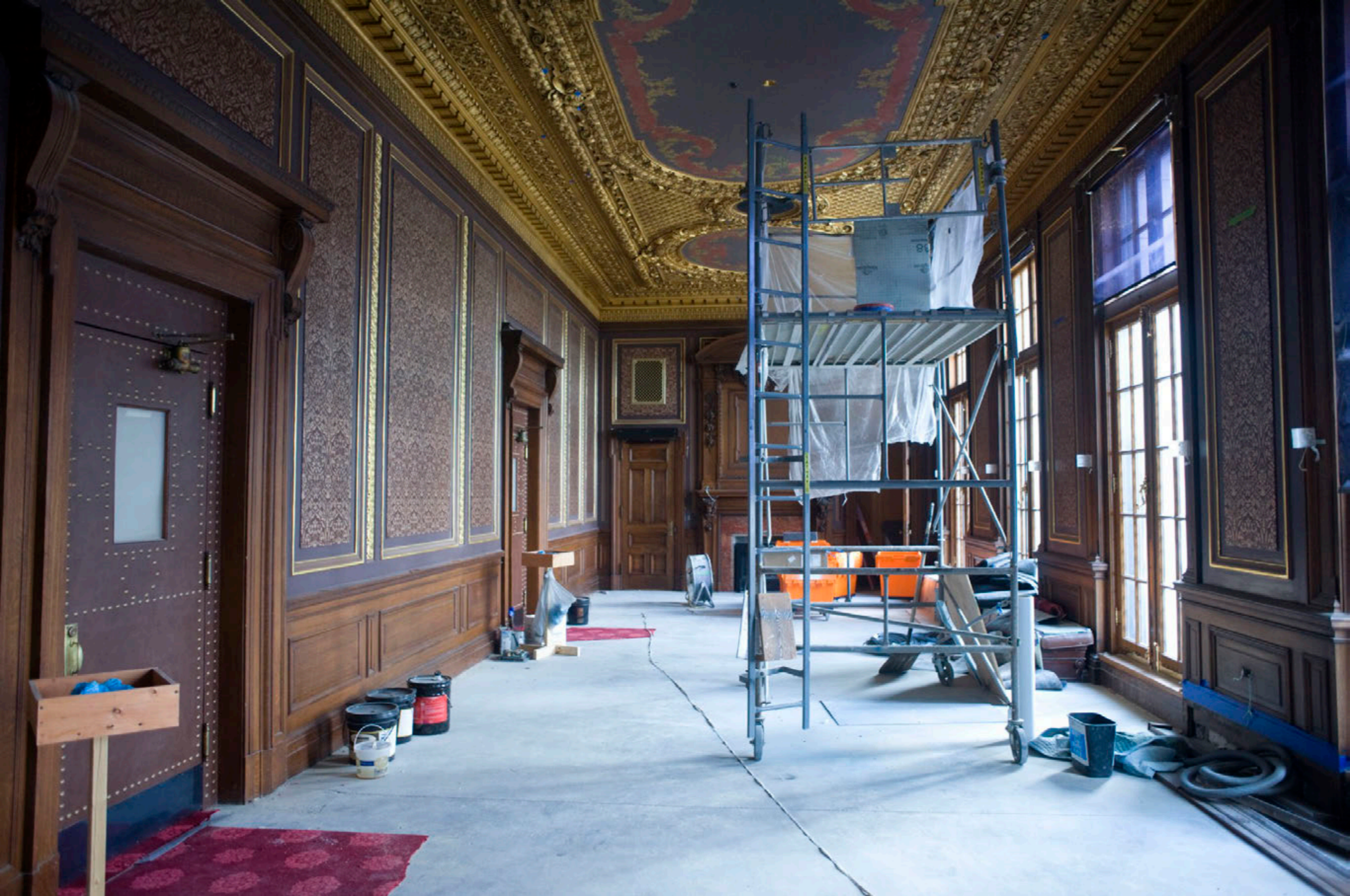
Senate Chamber Retiring Room being Restored. This is a room only used by Senators. The Public and even House members are not allowed in it by Senate Rules.
