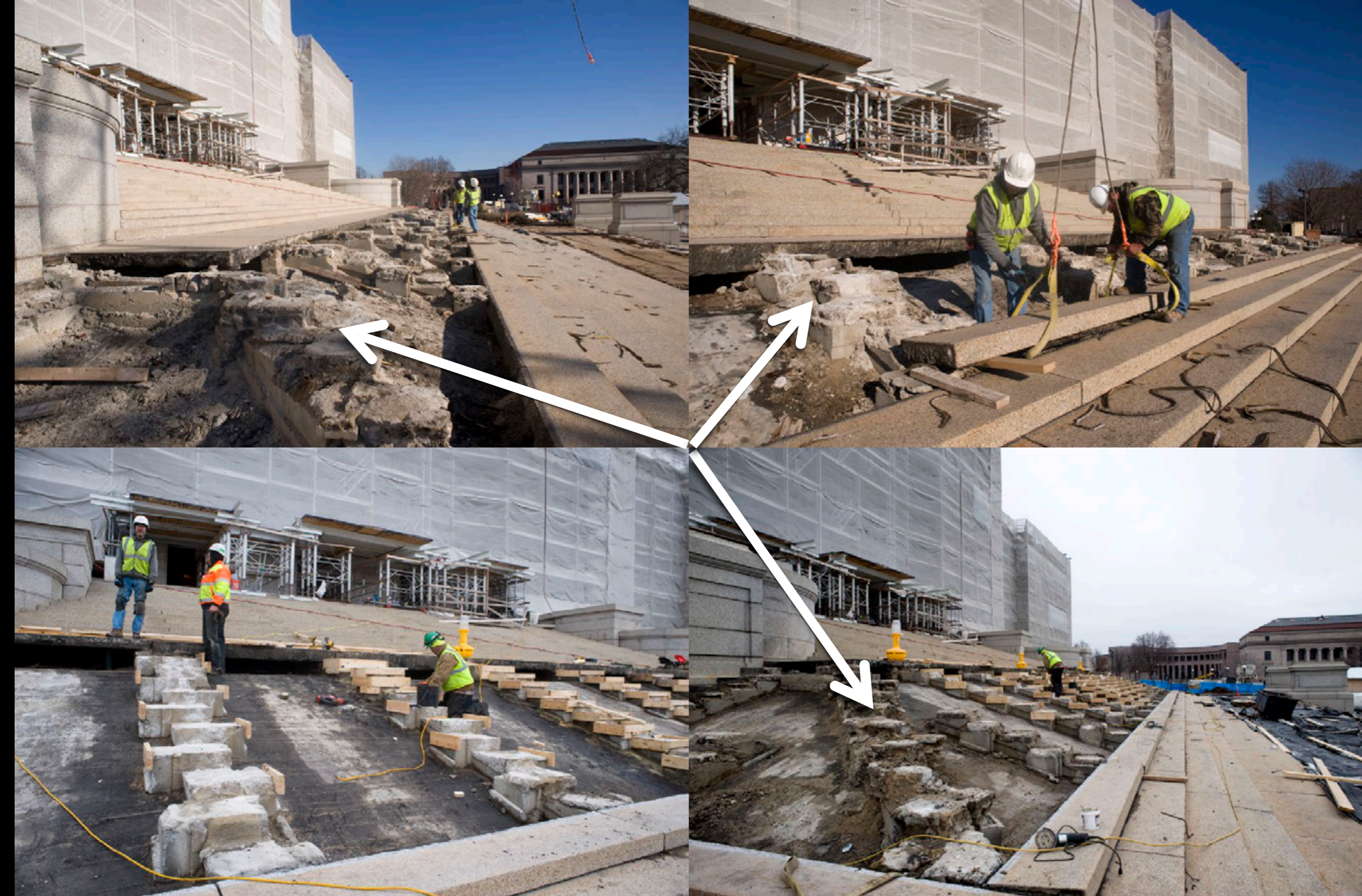
Granite steps in front of Capitol needed repairs, replacement and resetting. The foundations under the steps were crumbling. This was an additional $22 million cost that was discovered during the foundation restoration of the Capitol.
