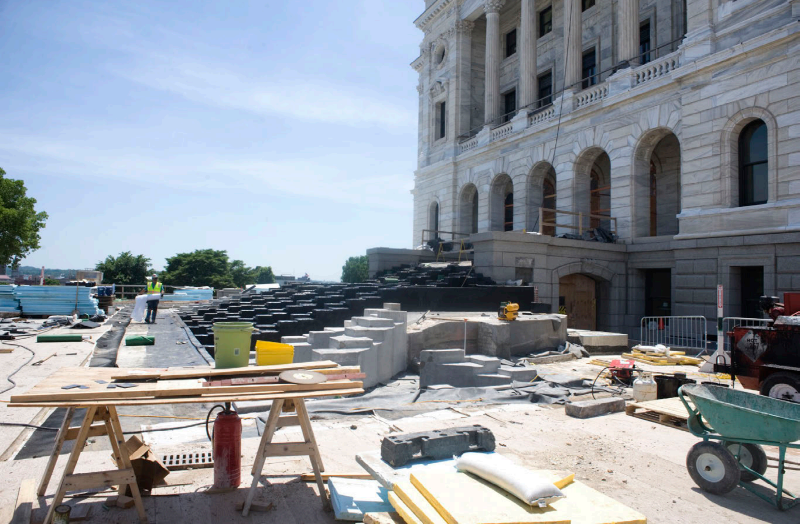
All of the granite step foundations of Capitol had to have their granite steps reset, repaired and replaced. The Supreme Court wing steps of the Capitol are being rebuilt above.
