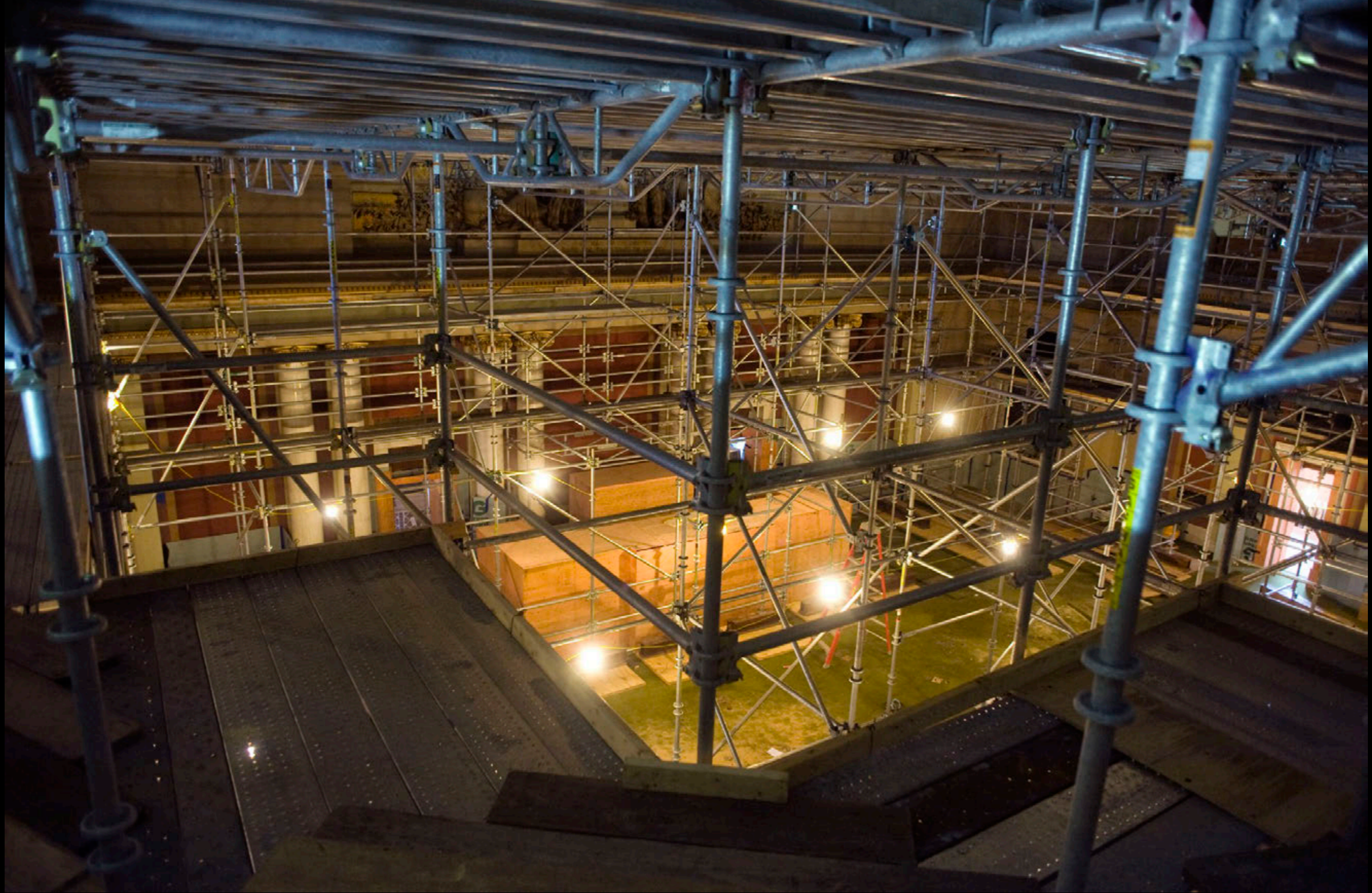
Scaffolding fills the House Chamber. The Speakers Rostrum is covered in protective sheets of particle board.
