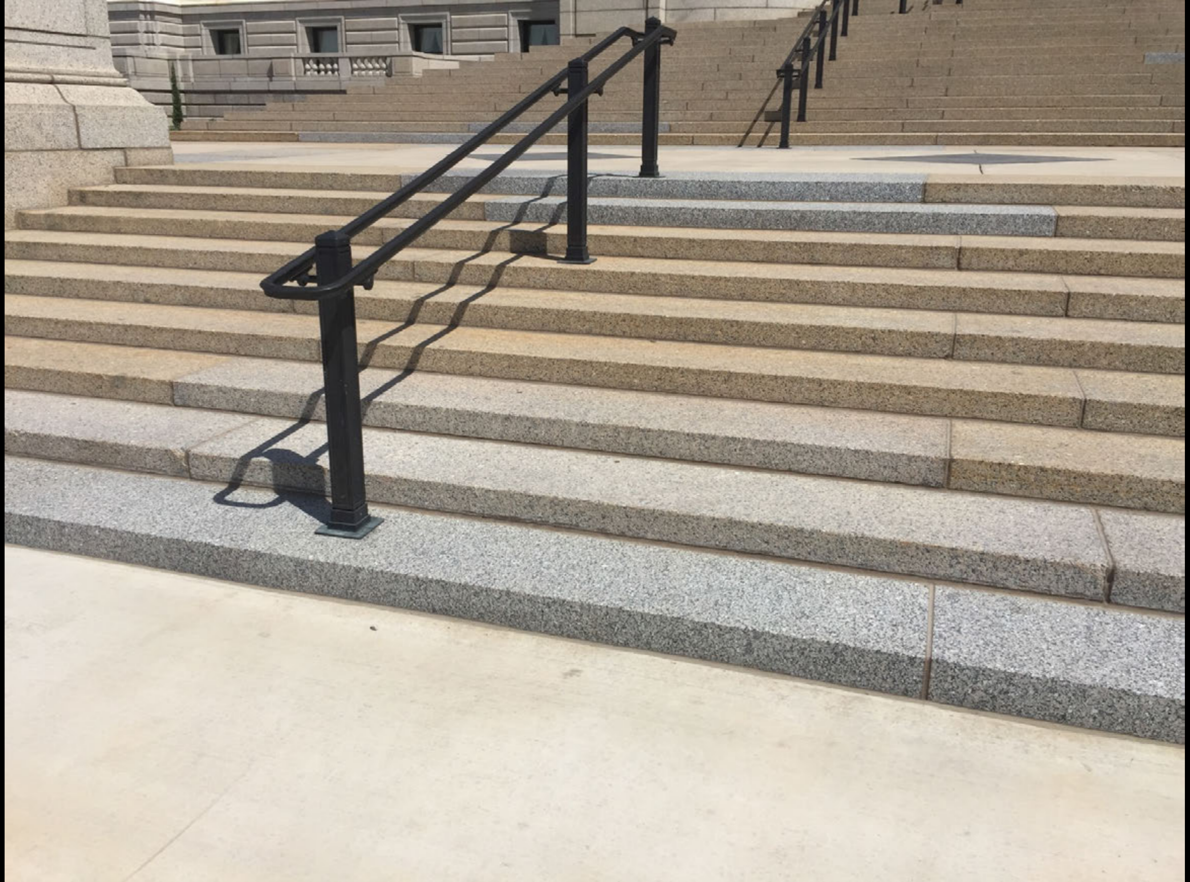
New Granite Steps in front of the Capitol show contrast in the replacement, lighter colored granite. June 2017
