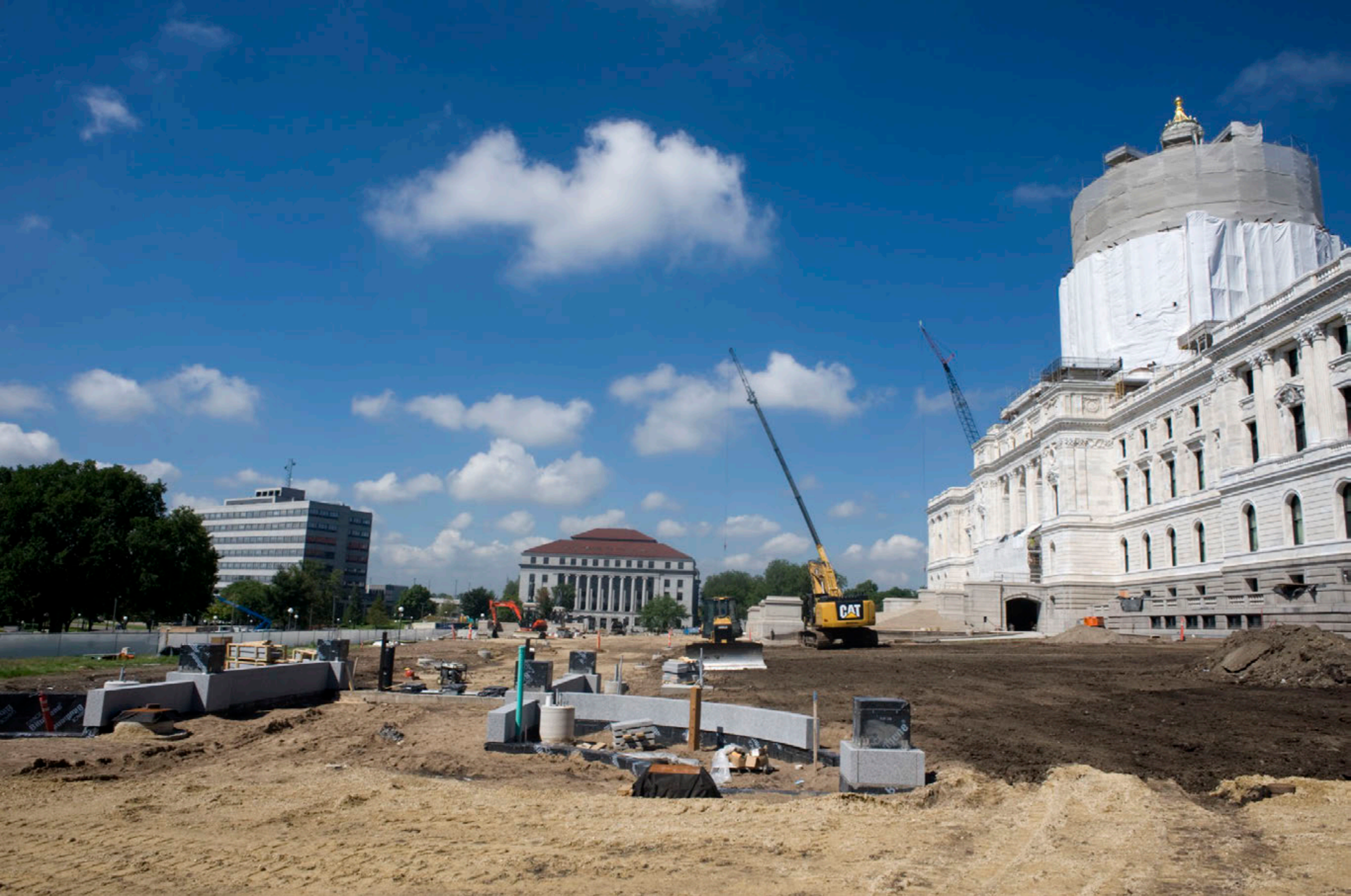
The entrance to the new Capitol Mall on the Judicial Building's side takes shape. Looking from the Judicial Building to the State Office Building.
