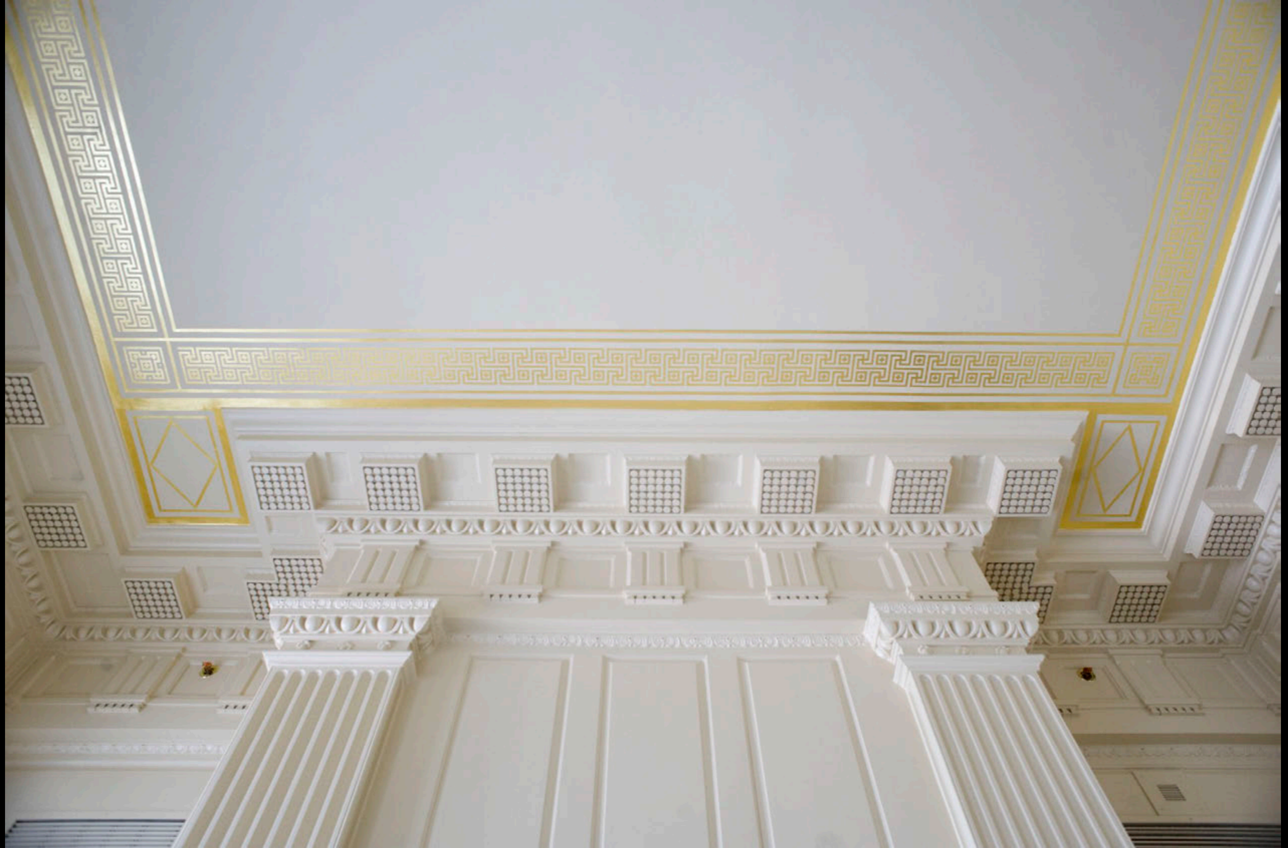
Supreme Court Retiring Room restored the original 1905 gold foil Greek fret design around the ceiling.
