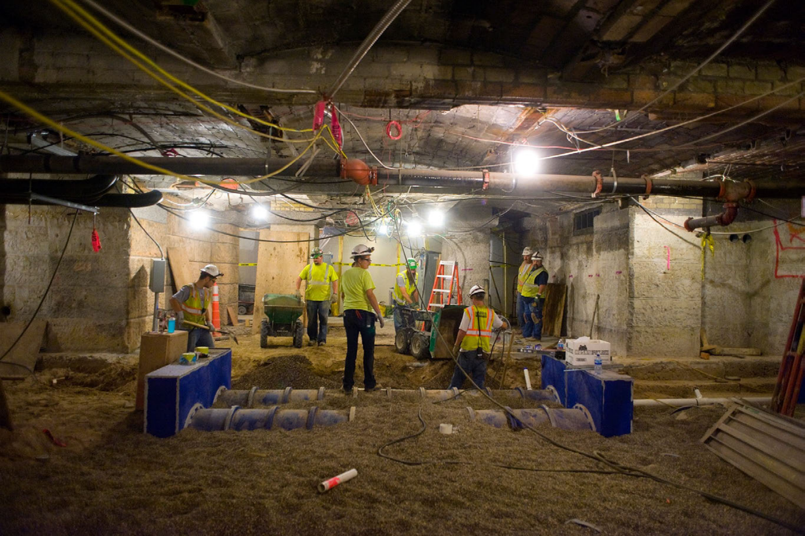
The lowest level of the Capitol. Never accessible except by maintenance. It now will become an impressive, new public space.
