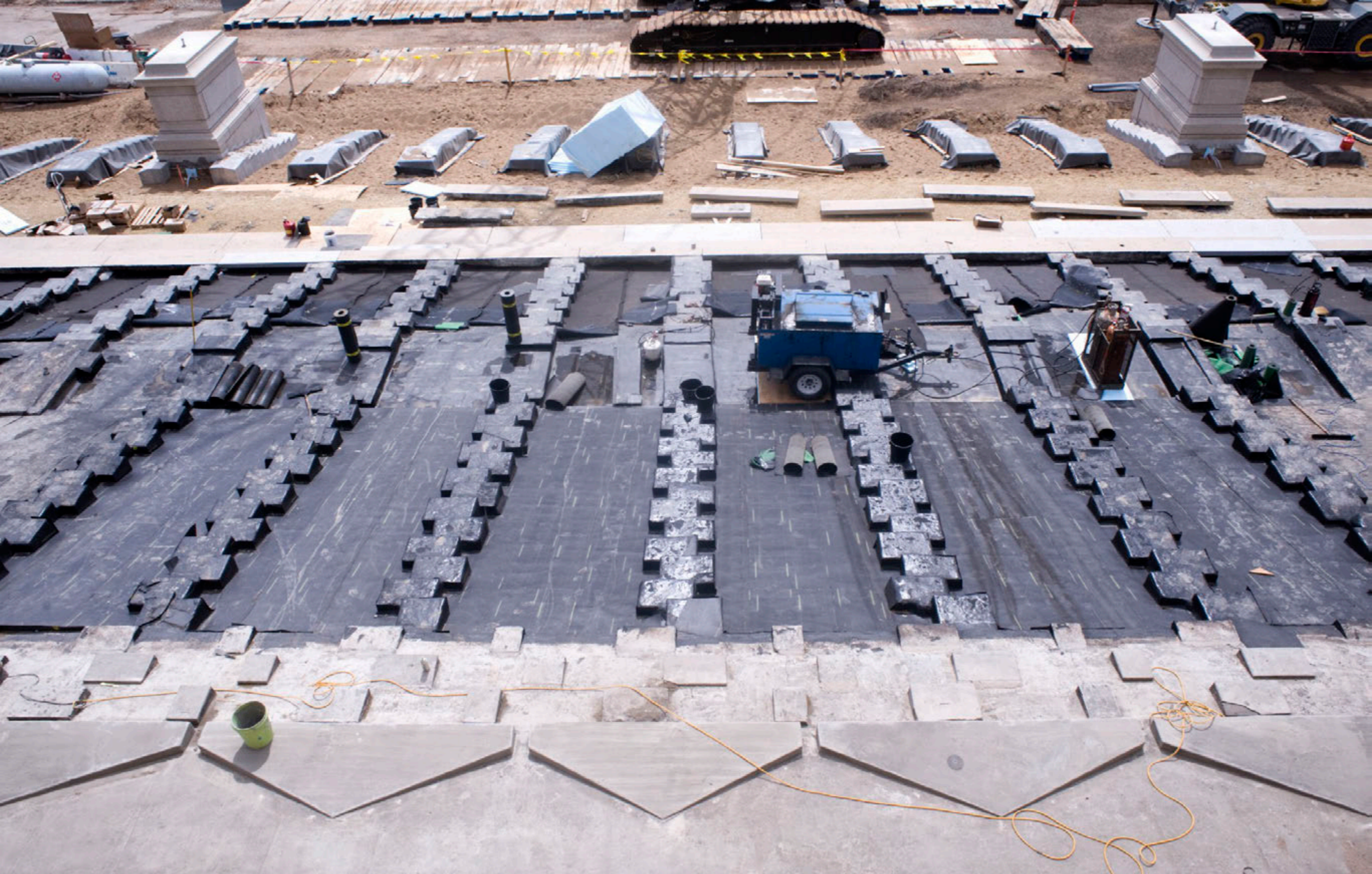
The granite step foundation in front of Capitol is now ready for the installation of the granite steps.
