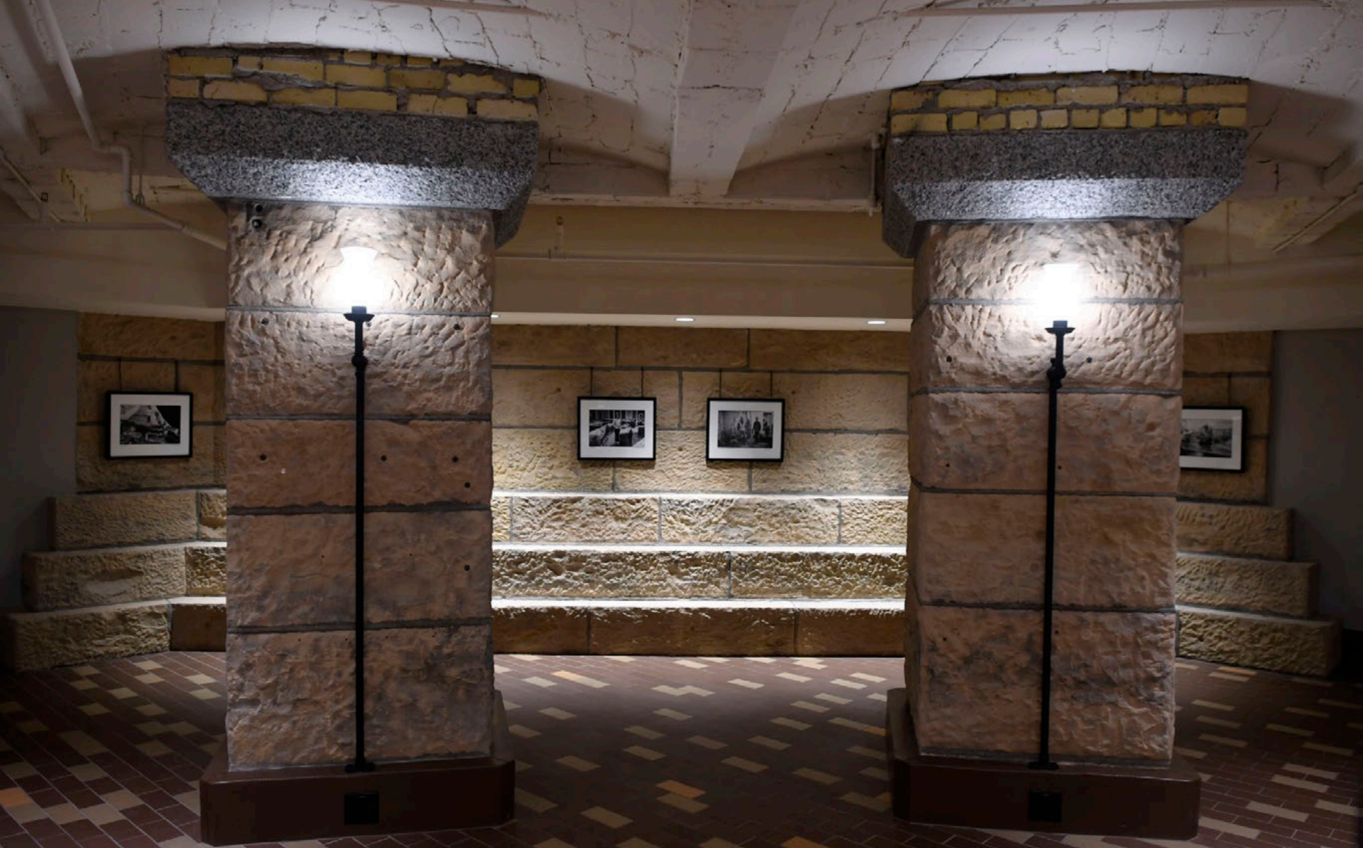
Tom Olmsheid pictures now adorn the walls that were buried in debris and expose the foundations of the Capitol.
