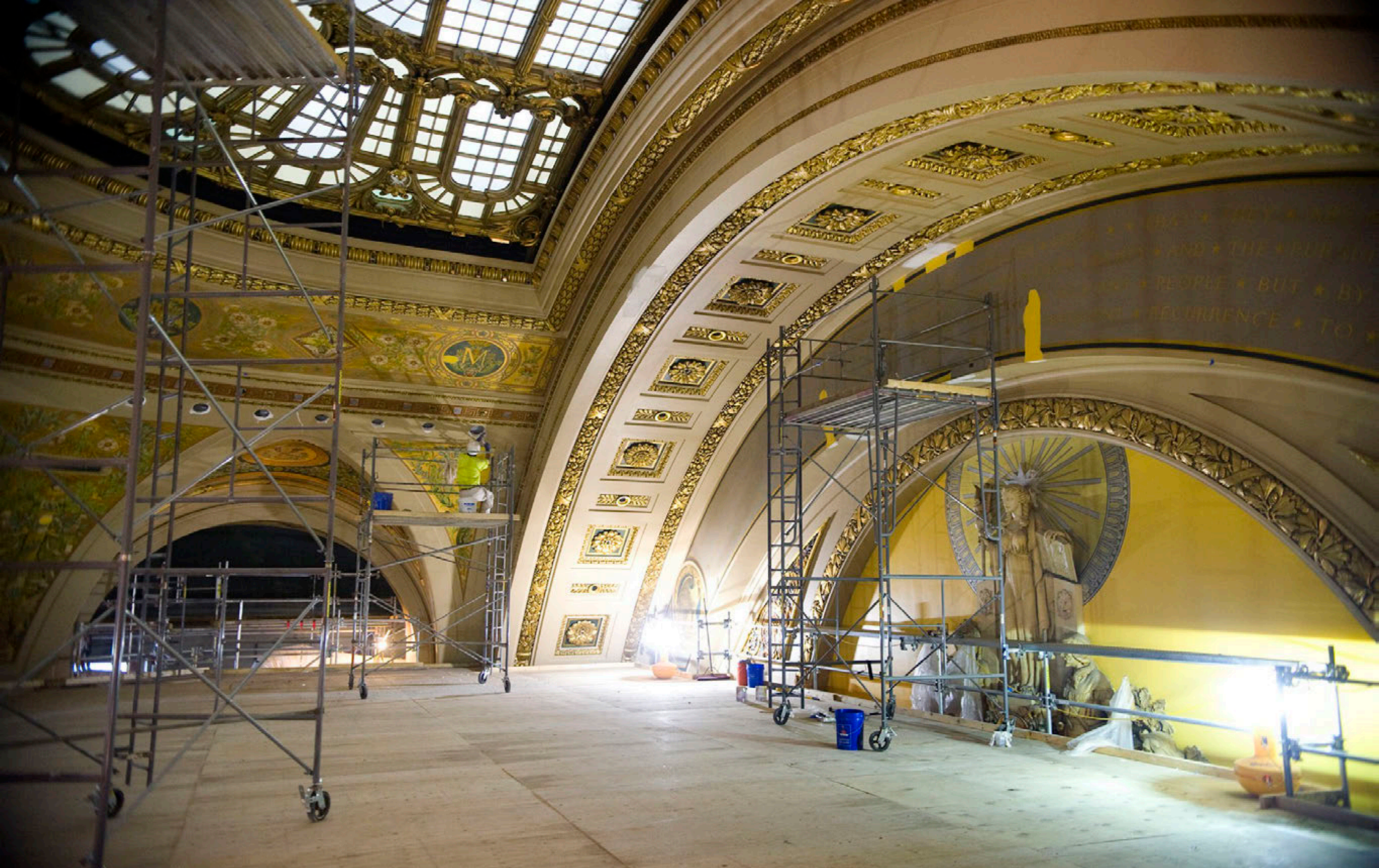
Scaffolding fills the upper most areas of the House Chamber to allow restoration of the sculpture and frescoes and skylight.
