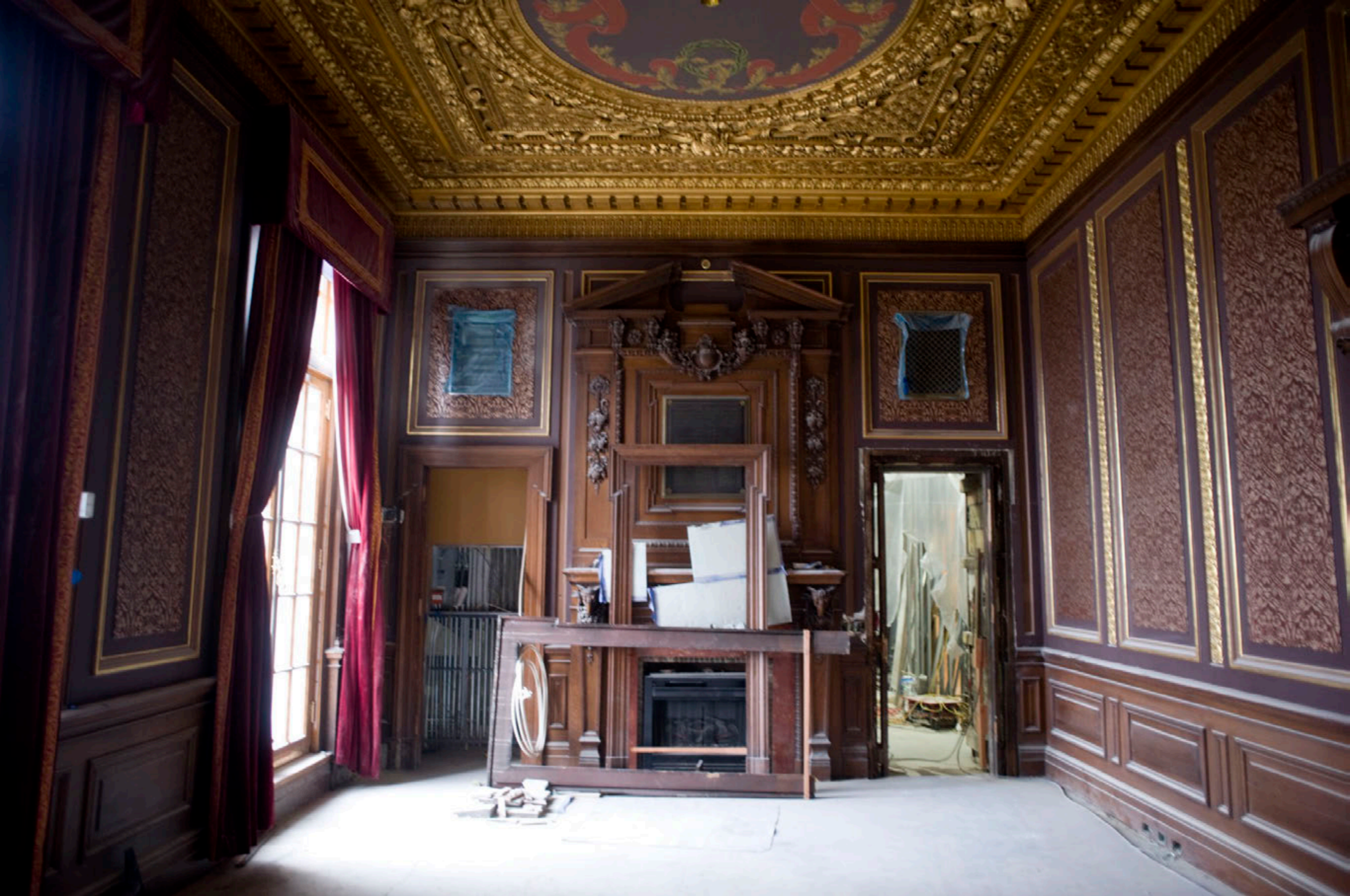
Senate Chamber Retiring Room being Restored. This is a room only used by Senators. The Public and even House members are not allowed in it by Senate Rules.
