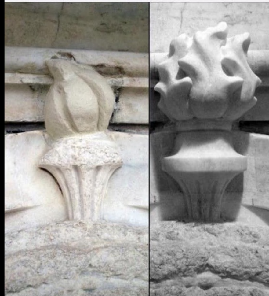
What a dramatic difference between the torch before the repair and after!
