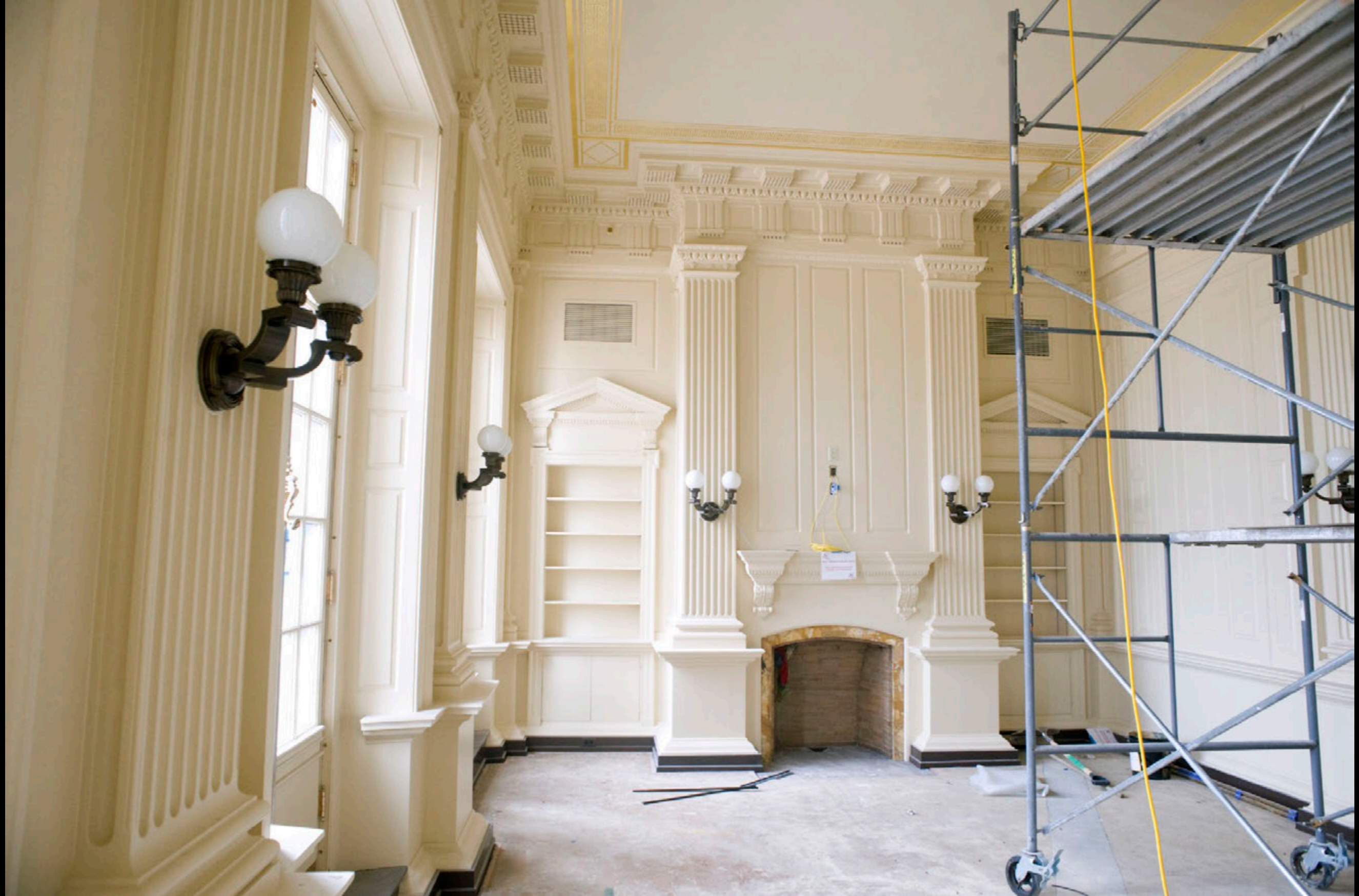
The Supreme Court Retiring Room was repainted with the original colored paint. Light fixtures restored to original design.
