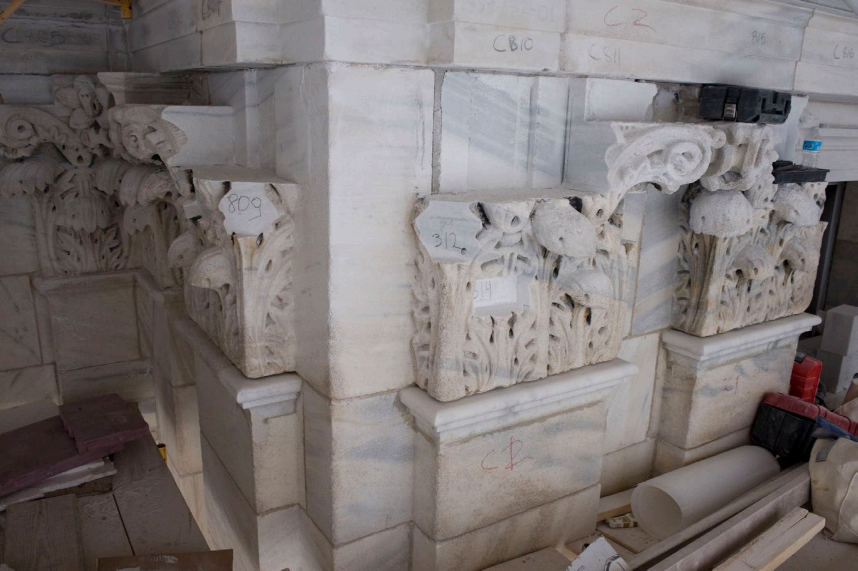
Damaged marble sections are cut away to be replaced by restored marble sections.
