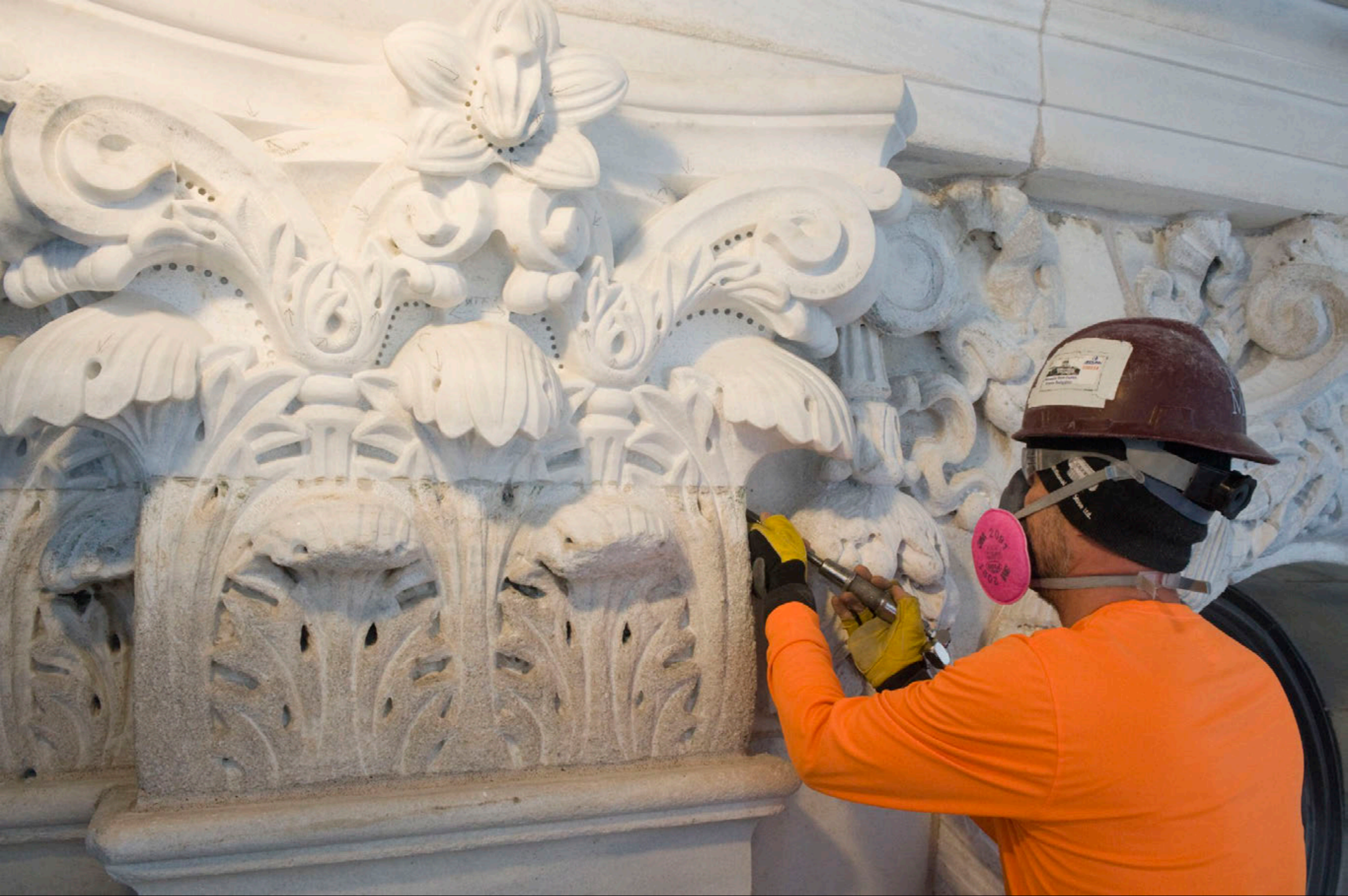
Contrast between capital restored marble sections and original marble sections are dramatic.
