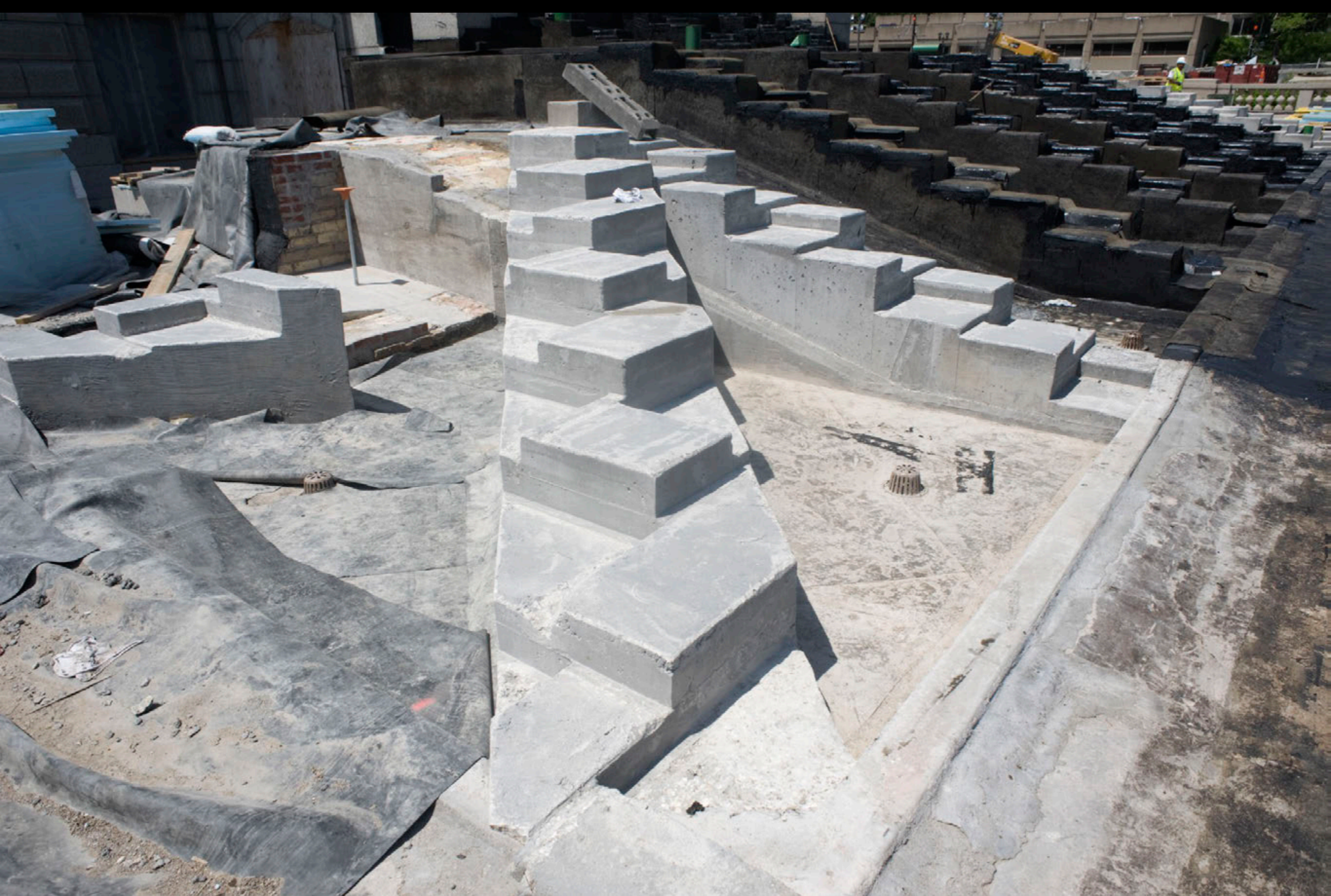
All of the granite step foundations of Capitol had to have their granite steps reset, repaired and replaced. The Supreme Court wing steps of the Capitol are being rebuilt above.
