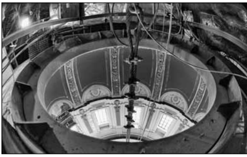
A metal ring has been installed in the top of the dome to allow hot air to rise into the frost dome. The hot air will then be mixed with cool air and exhausted out of the frost dome to outside the Capitol.
