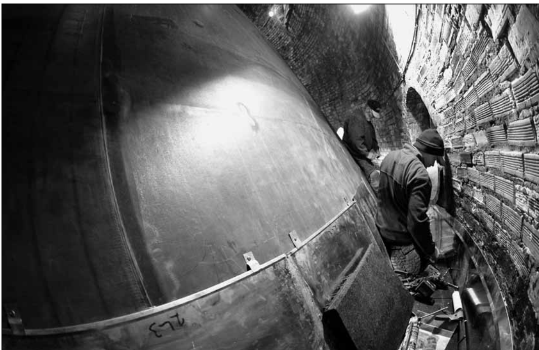
Greg Mathison, front, and Greg Christian of Innovative Building Concepts in Bloomington, install copper flashing at the base of the exterior of the frost dome.
